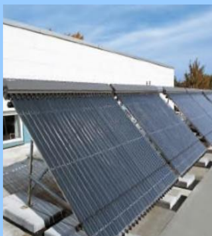
SOLAR THERMAL – HOT WATER
