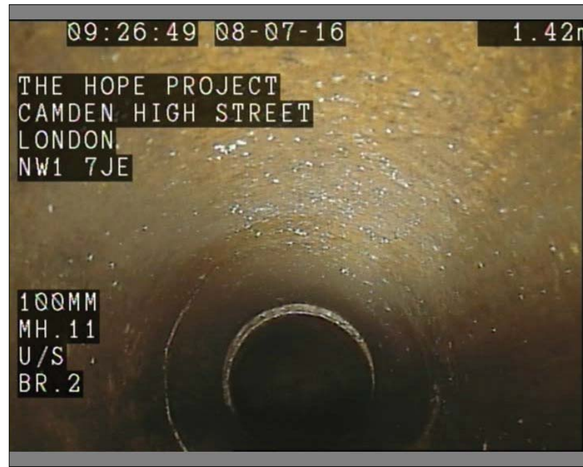
Photo: 26_26_163_A.JPG 1.42m, Crack, circumferential, from 7 to 5 o'clock
