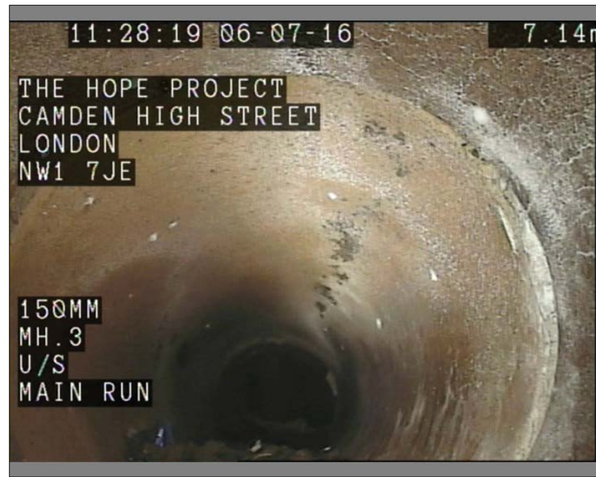
Photo: 13_13_70_A.JPG 7.14m, Settled deposits, coarse, 10% cross-sectional area loss
