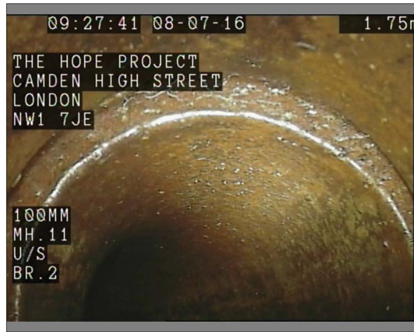
Photo: 26_26_164_A.JPG 1.75m, Crack, circumferential at joint, from 7 to 3 o'clock
