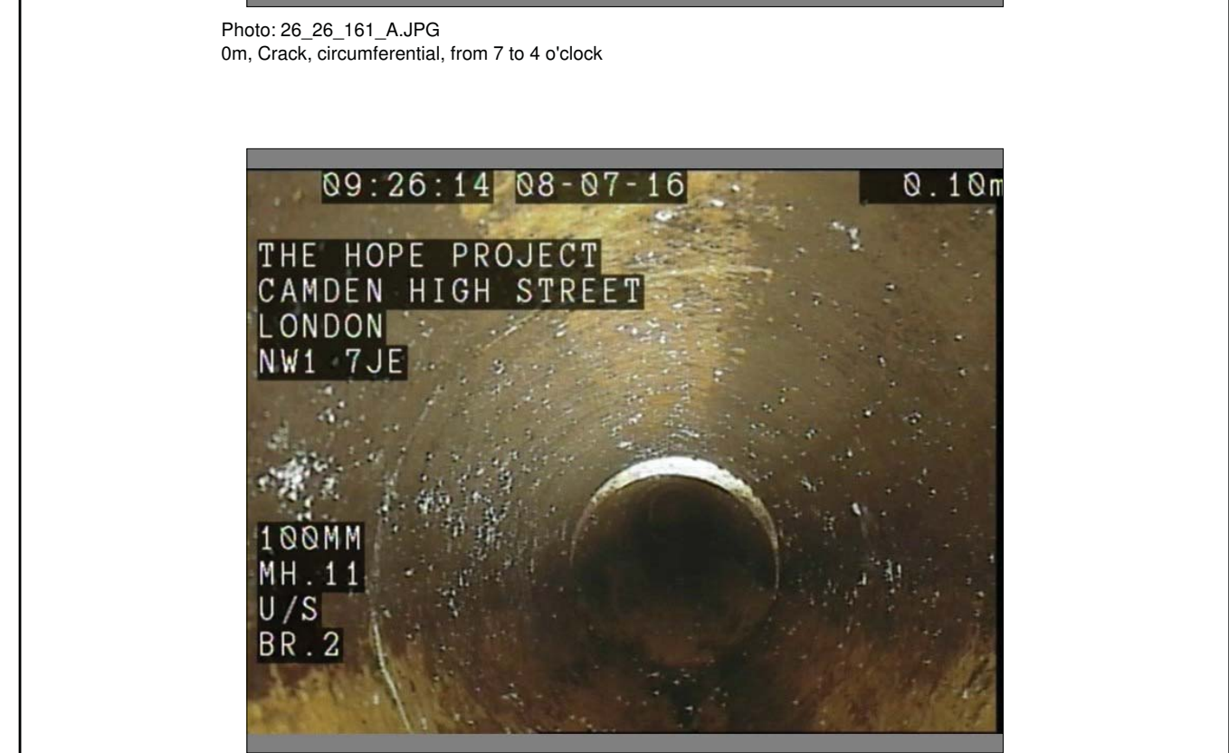
Photo: 26_26_162_A.JPG 0.1m, Crack, circumferential, from 7 to 12 o'clock
