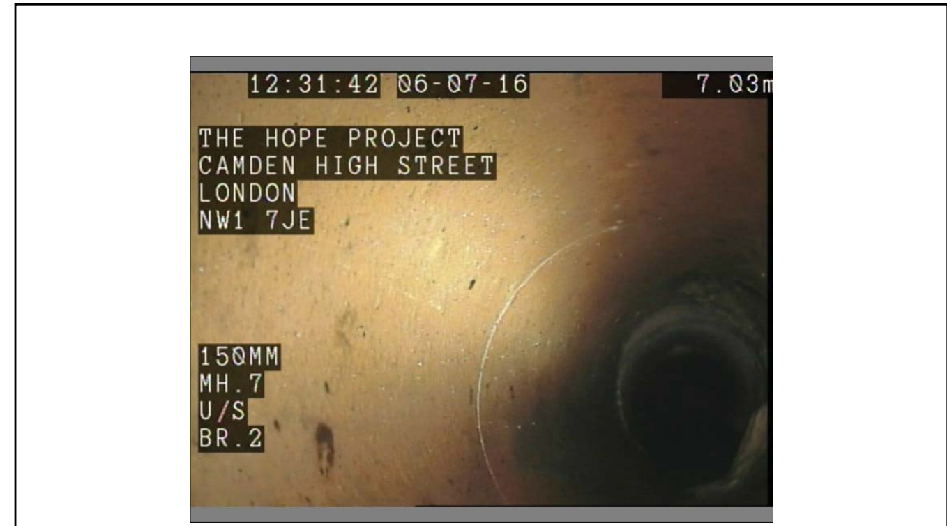
Photo: 20_20_129_A.JPG 7.03m, Crack, circumferential, from 7 to 11 o'clock
