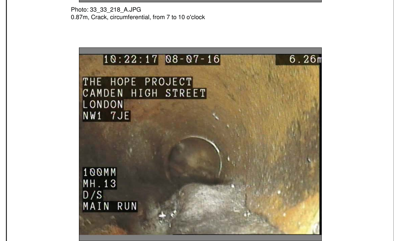
Photo: 33_33_227_A.jpg 6.26m, Attached deposits, encrustation, from 4 to 6 o'clock, 20% cross-sectional area loss
