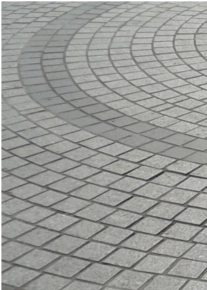
Sawn silver grey granite setts in stretcher bond
