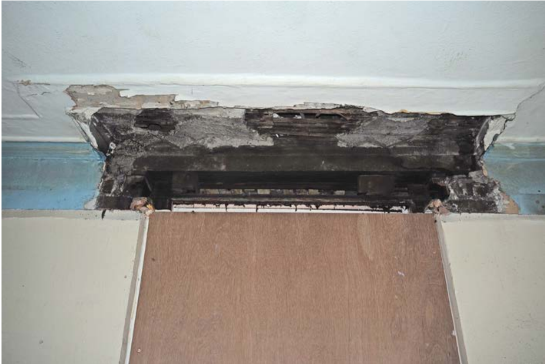
Evidence of shutter box and damaged cornice in the first-floor front room
