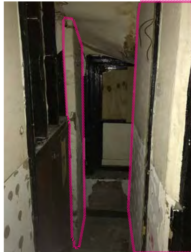
24 - Stair down to floor below. Original partition to secondary room visible on left-hand-side. Window on half landing boarded up
