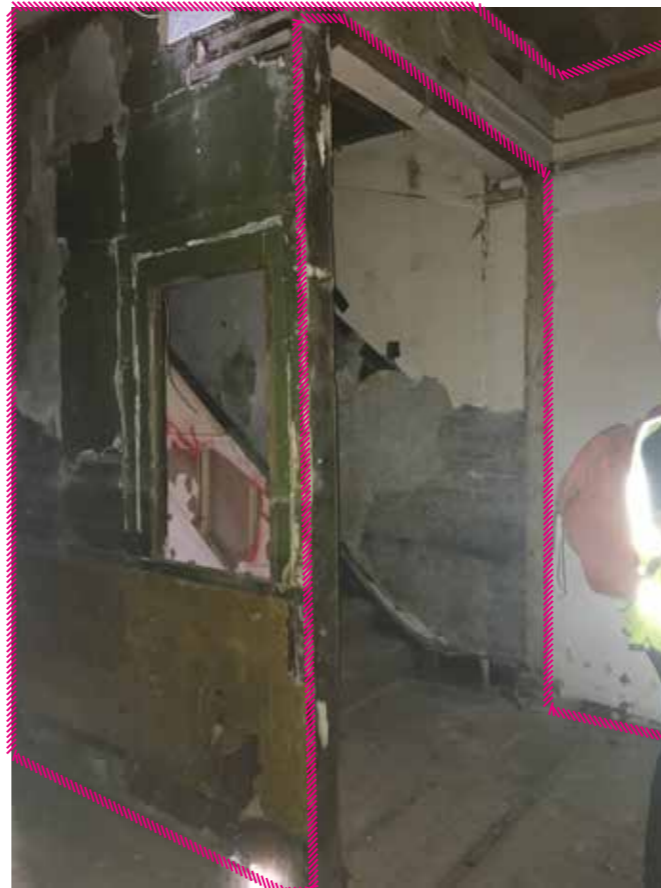
10 - Stair up to first floor. Original door opening partially boarded up and used as window.
