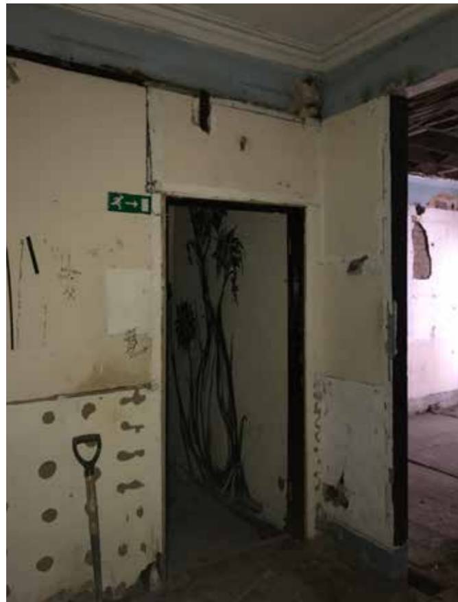
23 - Original door opening to rear room. Architrave missing. Original door opening to Primary room missing. Large opening linking primary and secondary rooms in original partition location.
