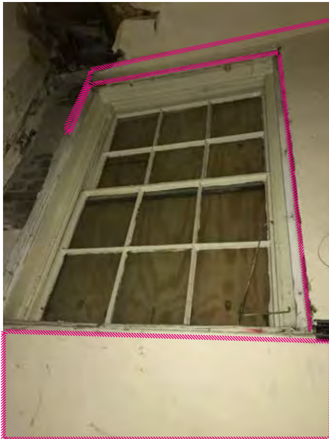
27 - Six over six sash window externally boarded up on half landing between first and second. Original architrave missing.
