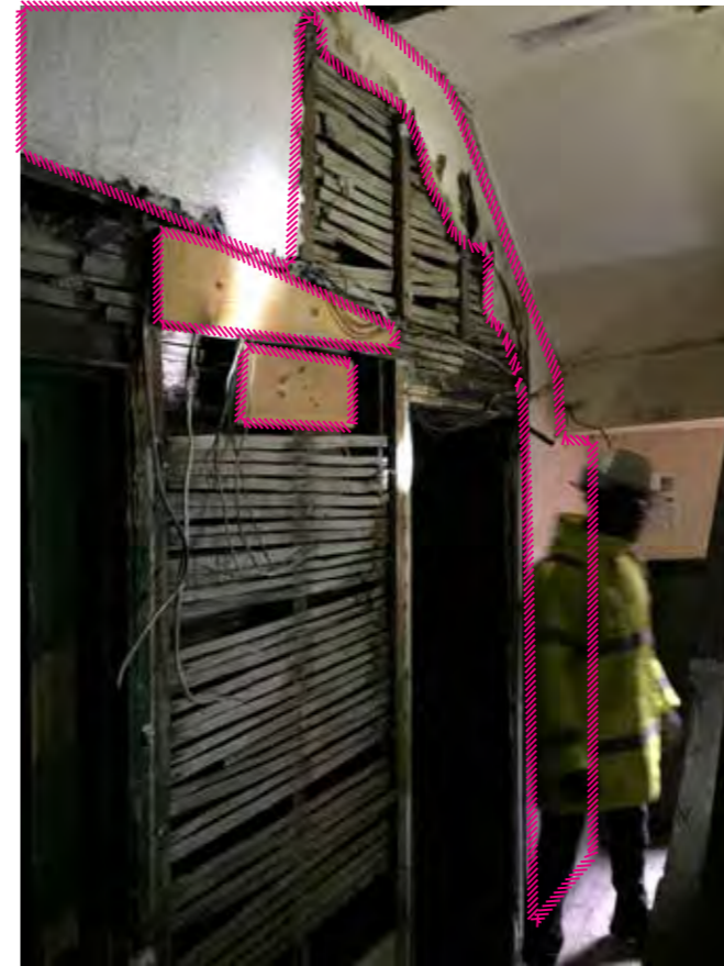
14 - Lathe and plaster stud wall in original position in stairwell, with new door opening
