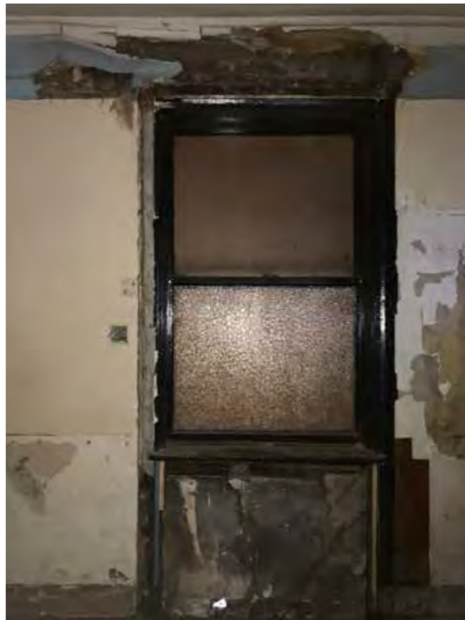
20 - Window in secondary room. Original cornicing damaged. No original architraves
