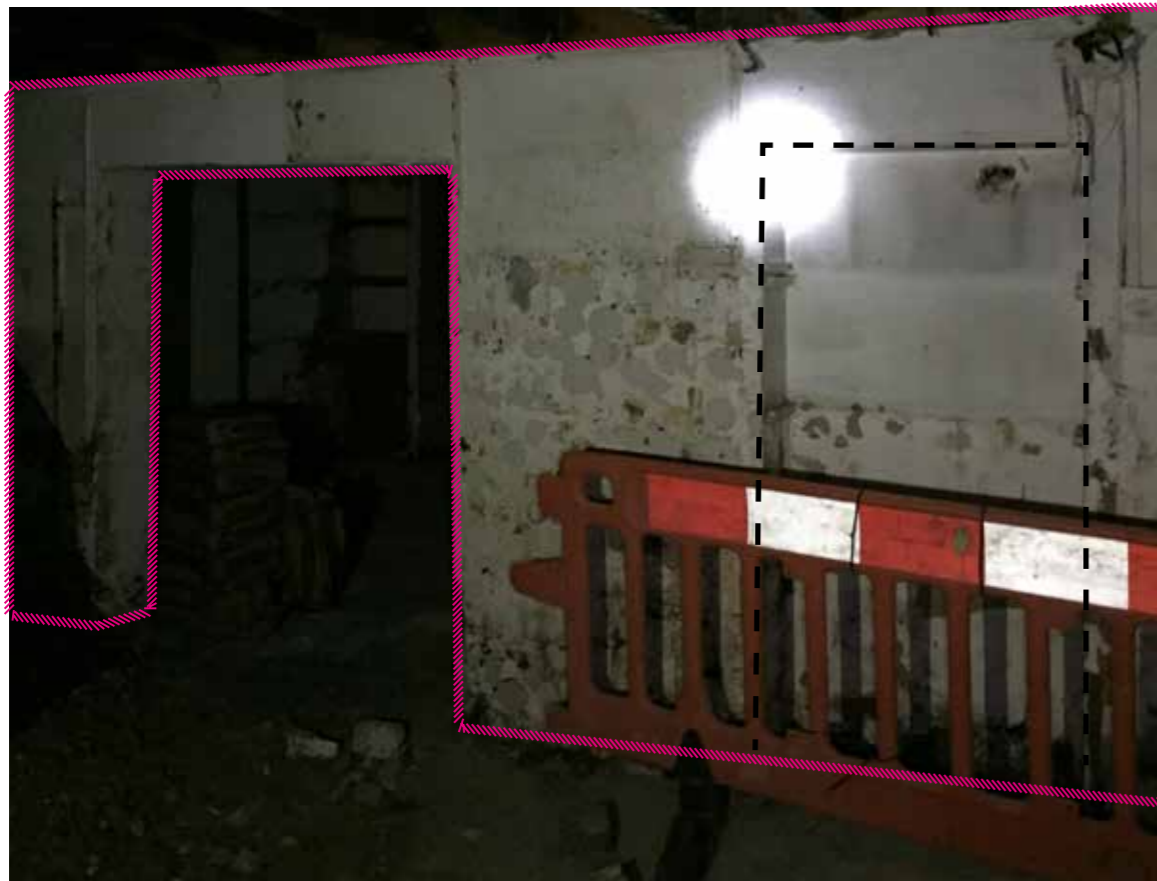
3 - Original opening from stair to primary room filled in. Lintols very low
