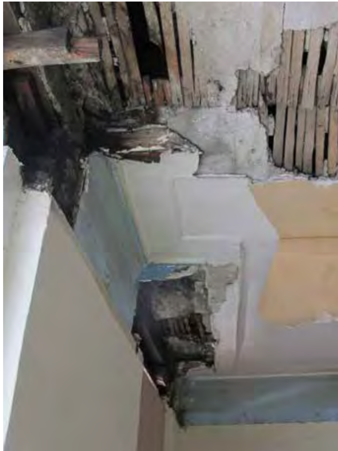
26.4 - Extent of remaining cornice line at first floor of 59 St Giles High Street . Also visible is the extent of the shutter box around the windows
