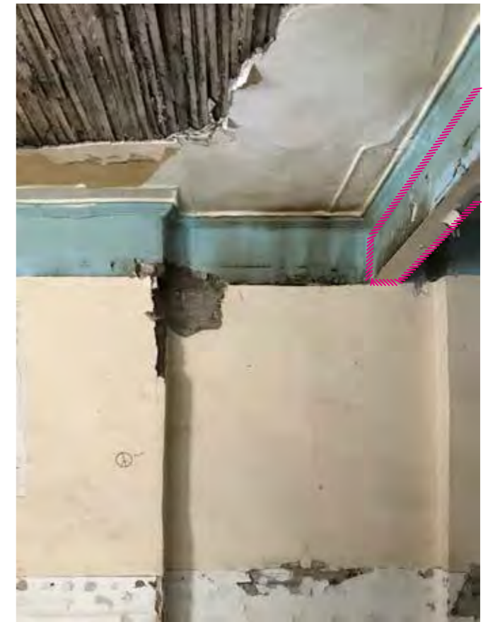
19 - Original corncing in front and rear rooms. Possible original timber beam holding joists above. Original chimney breast visible, opening boarded up.
