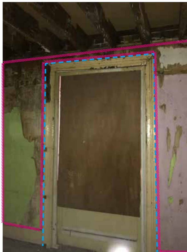
35 - Boarded up window and original architraves in secondary room. Exterior brick wall visible behind floor joists
