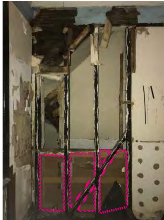
21 - Original partition between stair and rear room. Original cornicing damaged
