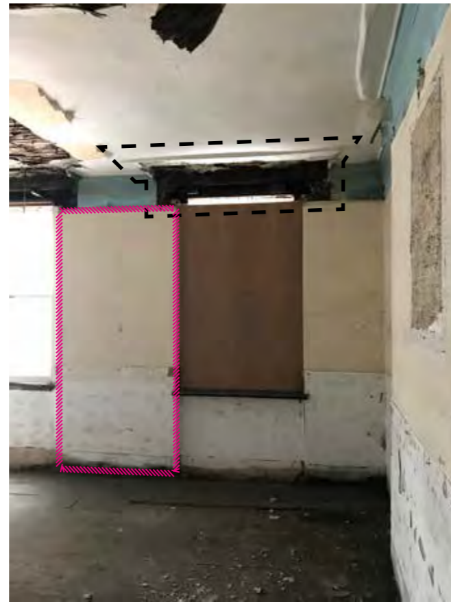
17 - Boarded window in primary room. Timber lintols exposed. Cornice line suggests original shutter box around windows.
