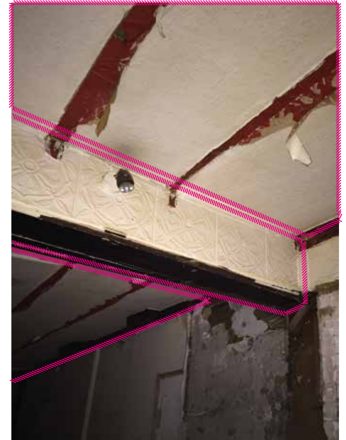
15 - Assumed steel beam boxed out at high level ground floor, on original partition line
