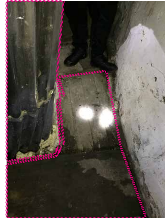
8 - Timber flooring soft underfoot and corrugated steel stuffed with foam to masonry wall in infill to the rear of the building.
