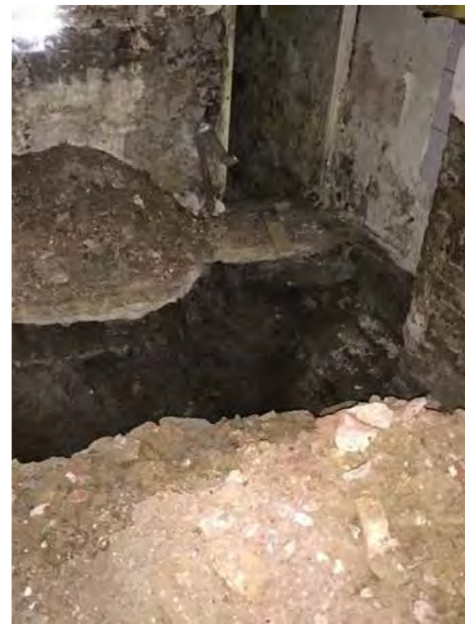
4 - Hole dug for UKPN works by Skanska Corbeled brick foundation visible adjacent chimney stack in primary room. Opening to area beneath St Giles High Street visible - currently inaccessible .
