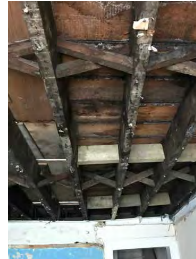
33 - floor joists at high level second floor primary room. New timber noggins visible to provide additional strength. Evidence of truncated floor boards on level above.
