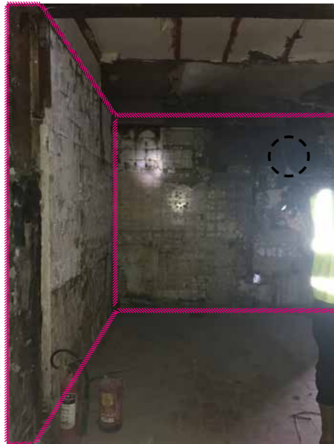
9 - Secondary room of ground floor. Extract duct visible in background.
