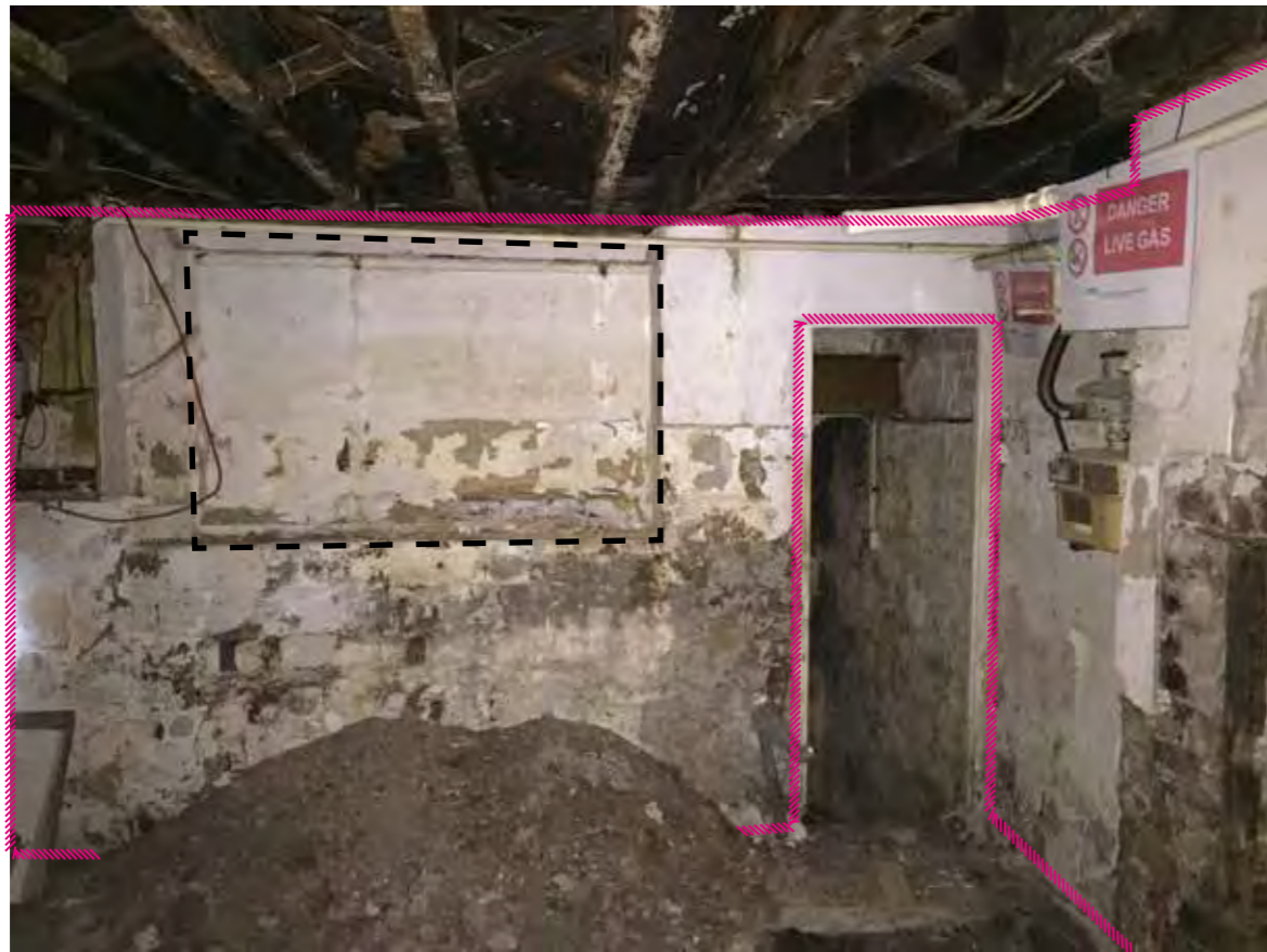
1 - Opening to area beneath St Giles High Street pavement - currently inaccessible. Note possible original window opening to street, filled in
