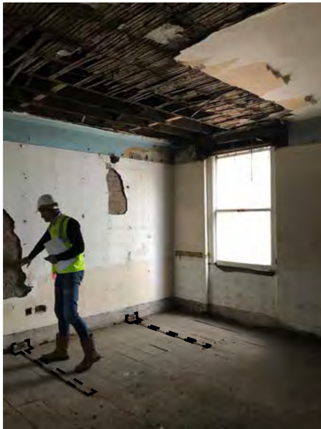
16 - Party wall strapping visible on timber floor. High level joists visible. Damage to window opening / cill visible.
