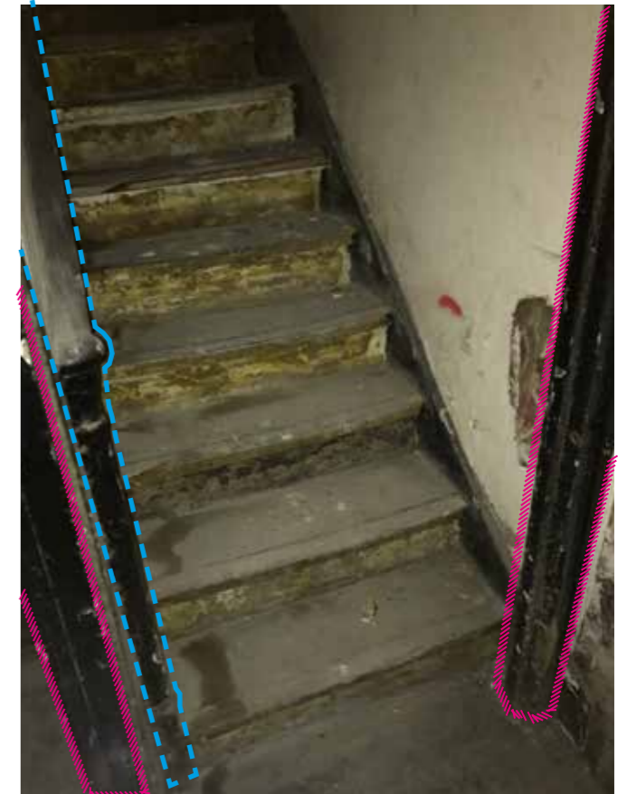
26 - Stair up to floor above. Possible original balustrade and knule post enclosed by partition?
