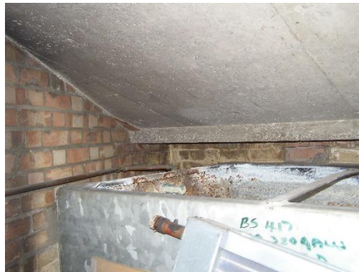
Internal water tank store
