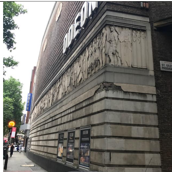
Damage to stonework of frieze
