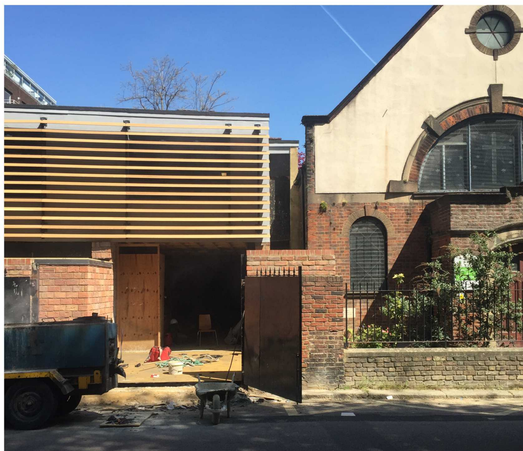
The Development Currently in Construction Adjoins to the Existing Church on our Proposed Development Site
