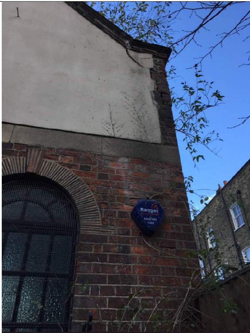
Plate 3: Crack along facias and brick.
