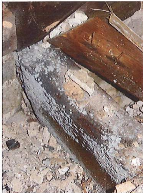
Spores on 3 rd floor timber beam which was showing signs of water staining
