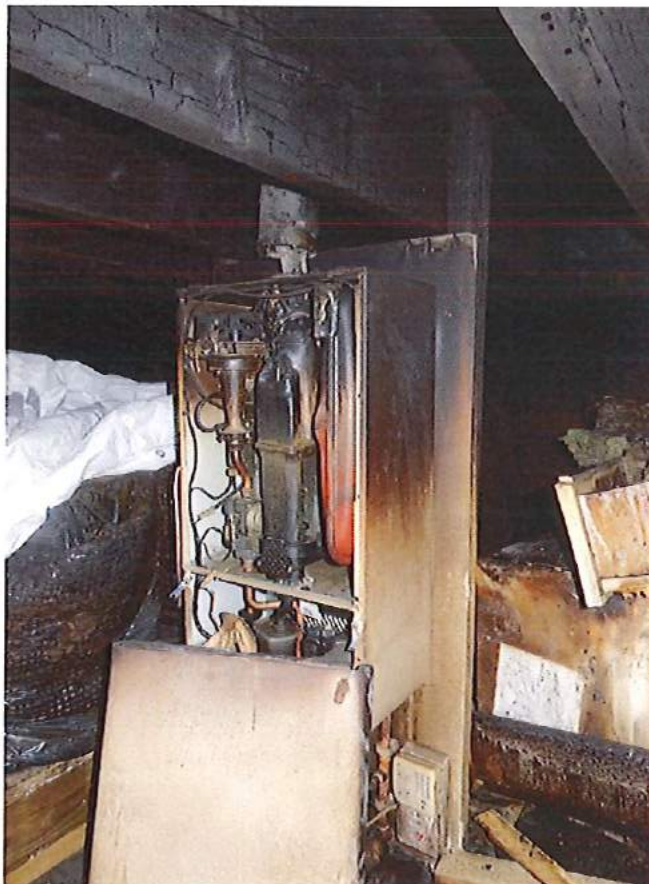
Boiler in roof space
