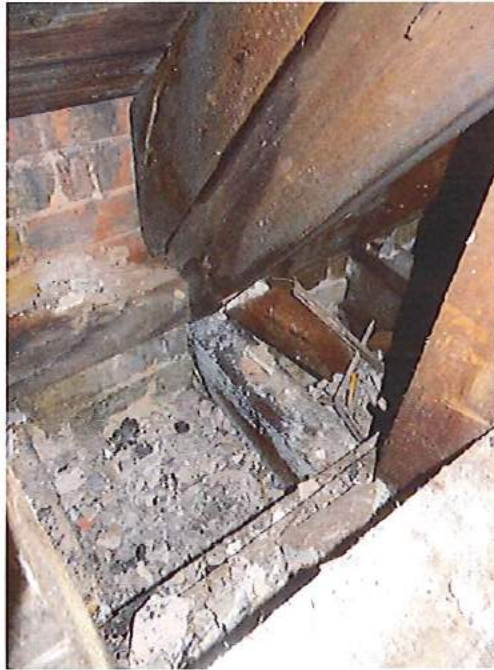
Water staining to rafters in vicinity of north dormer window
