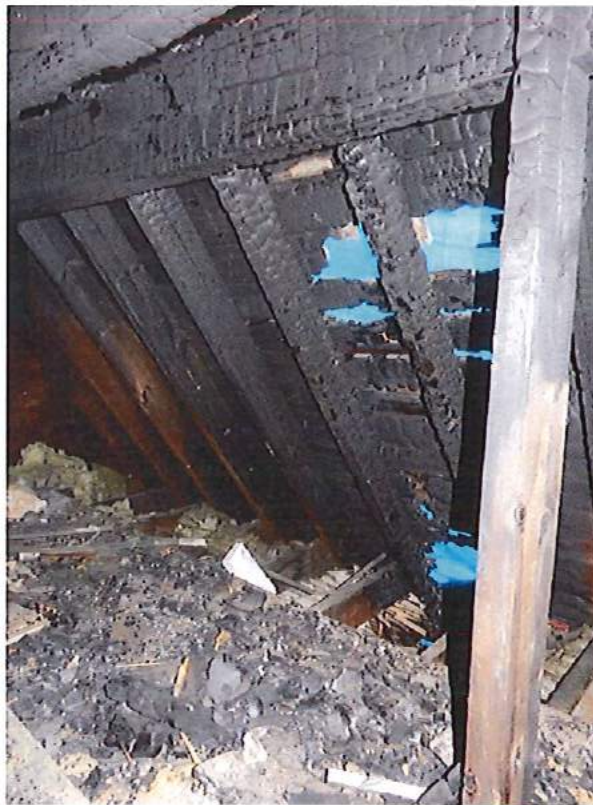
Badly damaged rafters plus sarking boards above dormer window
