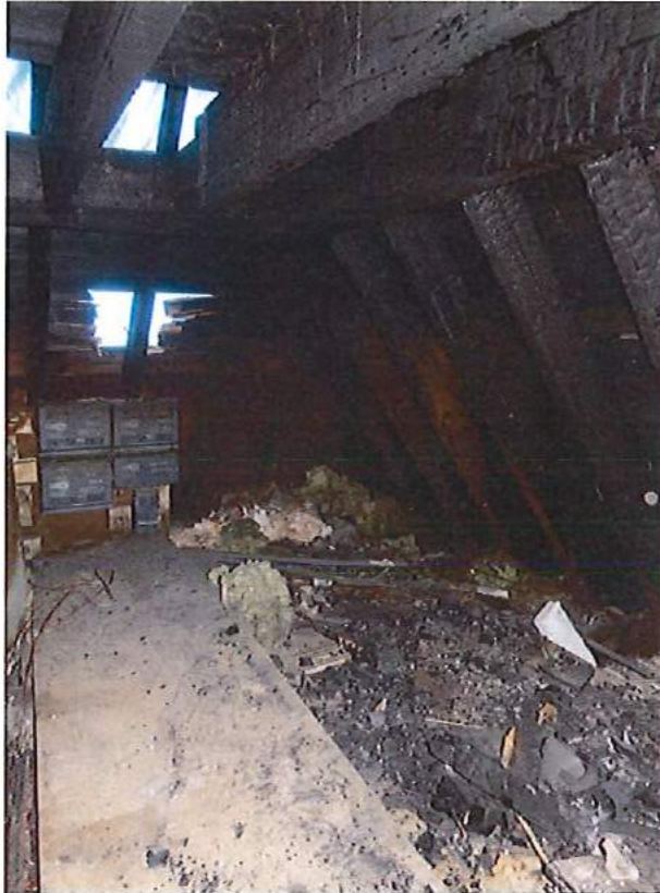
Further view of fire damaged roof section
