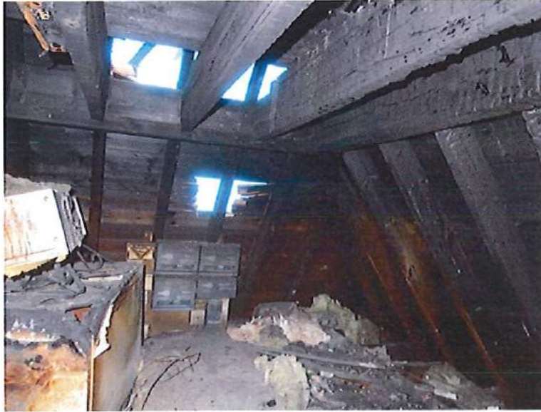
Badly charred rafter beams plus joists to the flat roof
