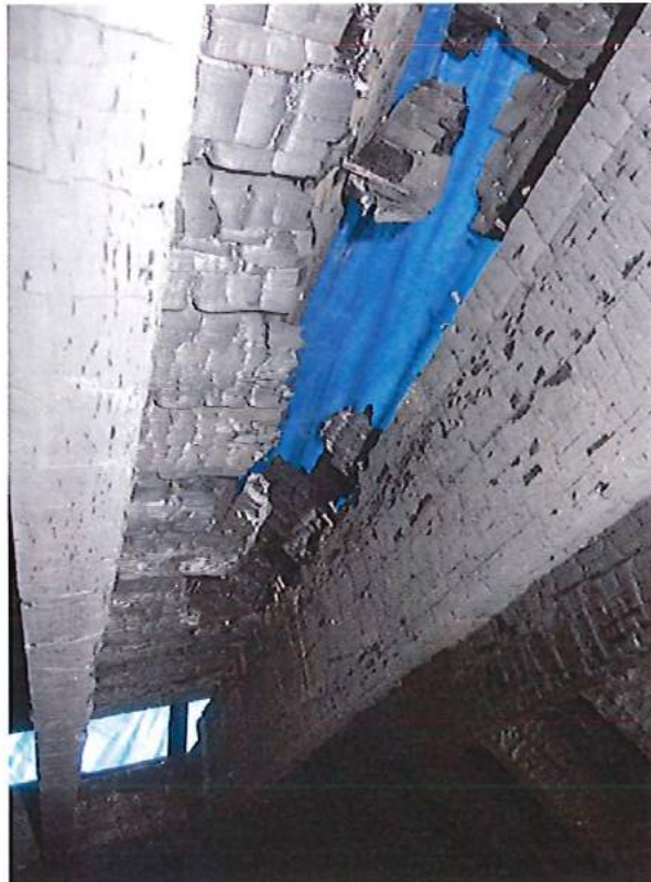
Heavily charred joists to the flat roof section plus sarking boards burnt thro' locally
