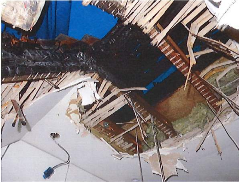
The north dormer window construction is also heavily damaged
