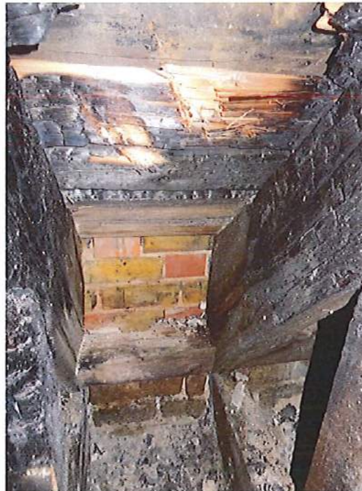
Fire damage to rafters extending down to timber wall plate at third floor level
