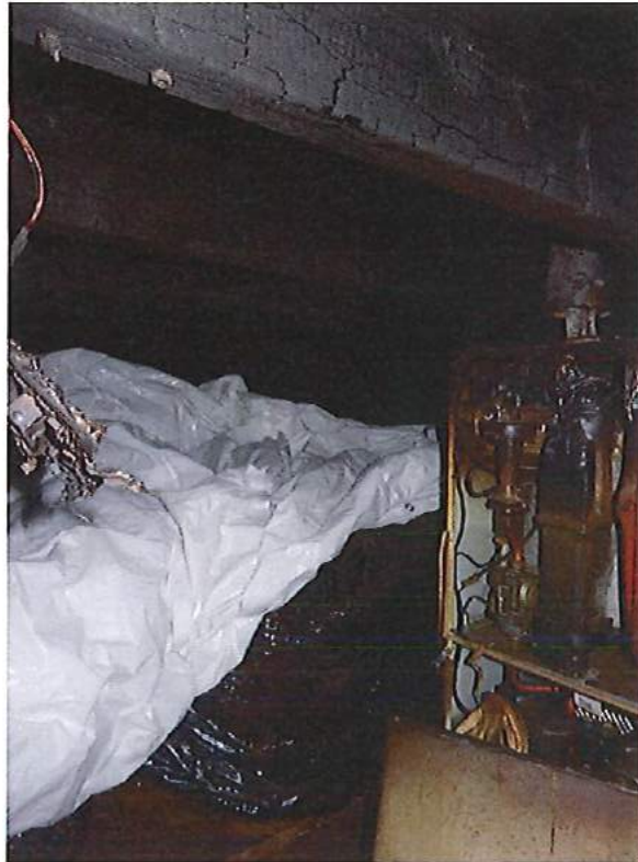
Lagged water tanks in roof space
