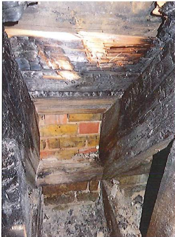
Charring of rafters down to third floor wall plate
