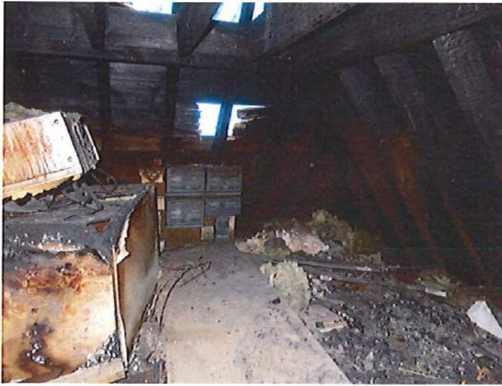
Stored goods and floorboards in roof space
