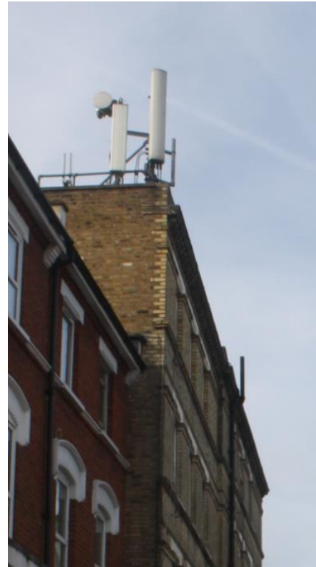
ANTENNAE ON ROOF OF APPLICATION SITE
