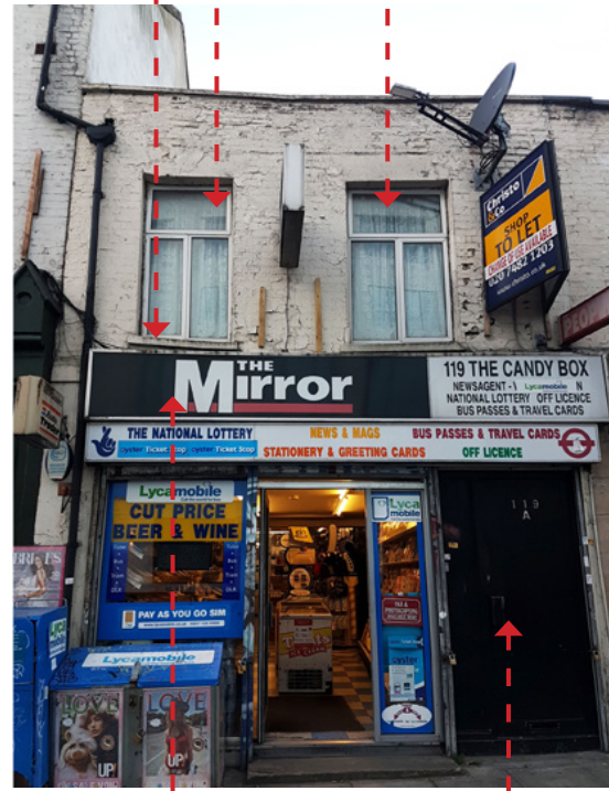
Existing signage/ shop front not aligned to Camden Planning Guidance Design (CPG1) section 7.10.
