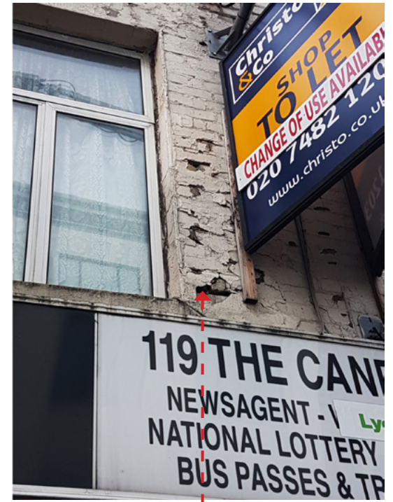
Painted brickwork peeling and mortar joints have become damaged
