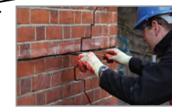
4. Using the HeliBar Insertion Tool, push one HeliBar into the grout to obtain good coverage
