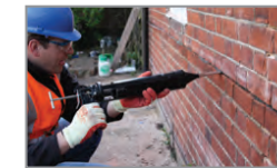
5. Insert a further bead of HeliBond over the exposed HeliBar, finishing 12mm from the face, and 'iron' firmly into the slot using the HeliBar Insertion Tool
