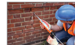
6. Re-point the mortar bed and make good the vertical crack with CrackBond TE3
