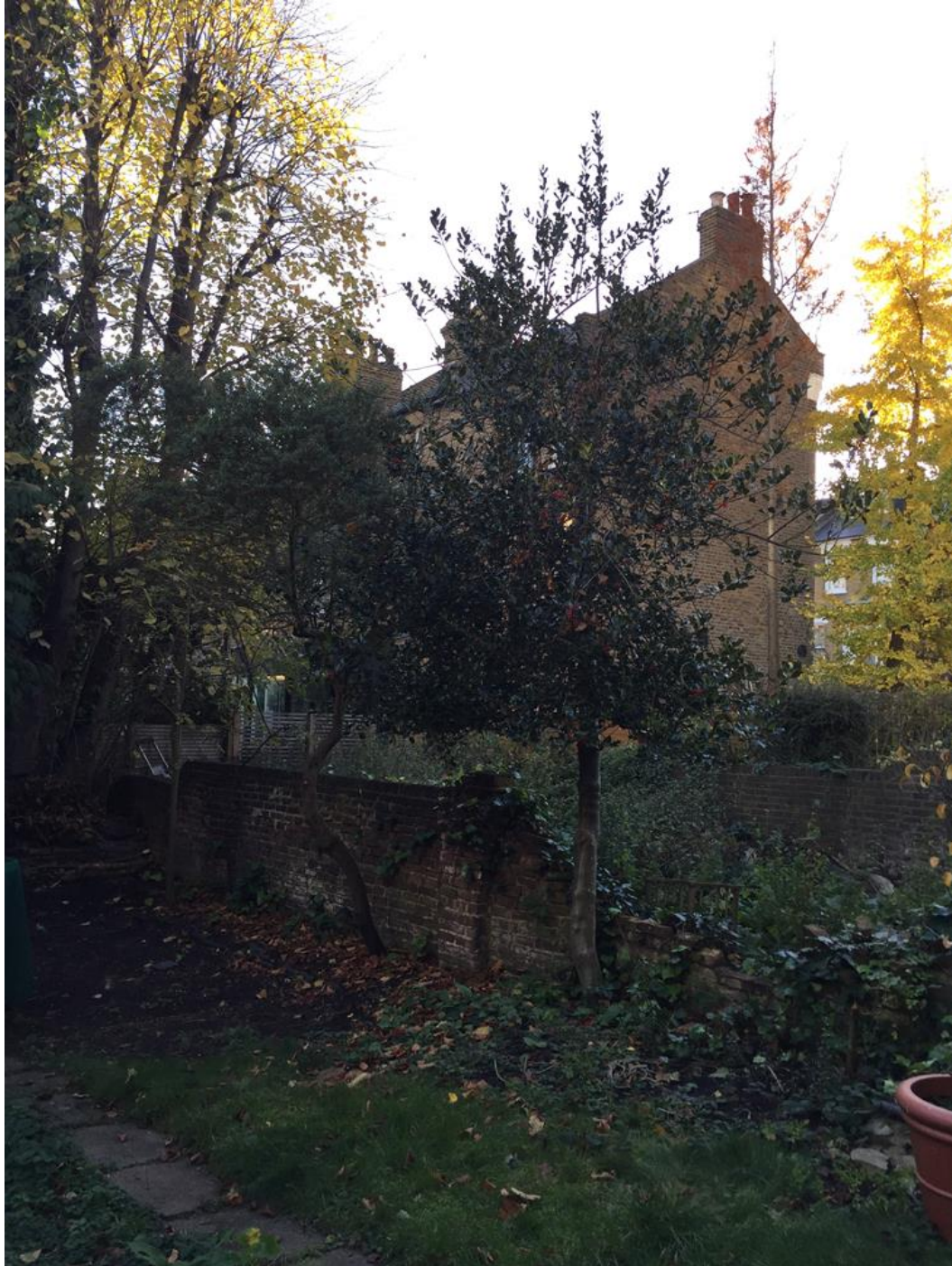
Photo 1. Holly (T4) in the centre (causing wall damage); Ceanothus (S3) to its left; and sapling Ash (T2) to the left of the Ceanothus.
