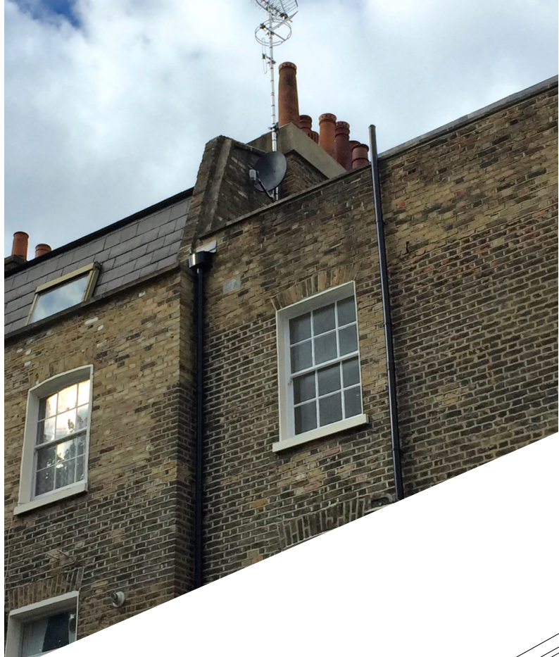
EXAMPLE OF IRS INSTALLATION - SATELLITE DISH (PAINTED BLACK), TV & RADIO AERIALS (at 33 FREDERICK STREET)
