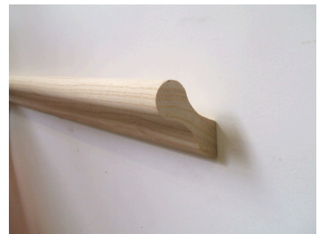
new pigs ear handrail installed once all furniture has been moved in (stripped stairs to remain unpainted)
