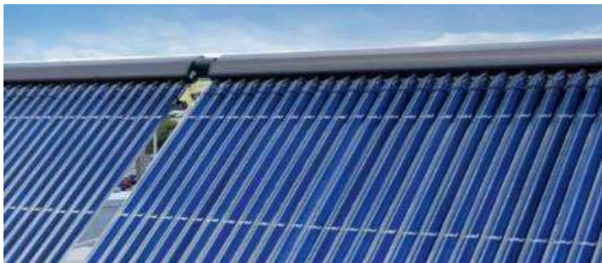
Figure 21. Image of an evacuated tubes solar thermal panel
