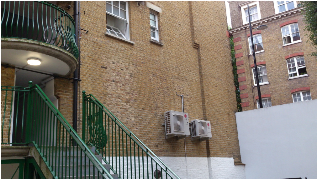
IMG-1 – Nearest Residential Façade And Installed Air Conditioning Condenser Units
