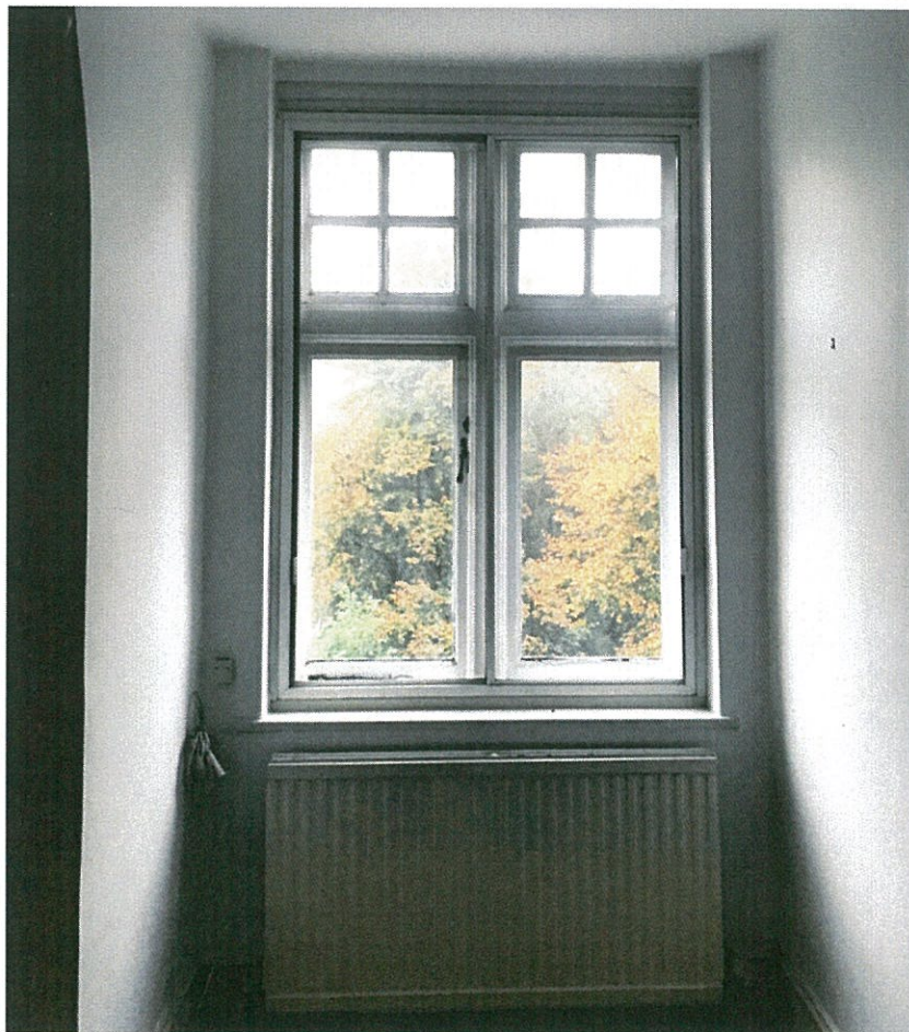
Image 4: The Pryors, Flat 27, typical casement window with top hung glazed lights and secondary glazing
