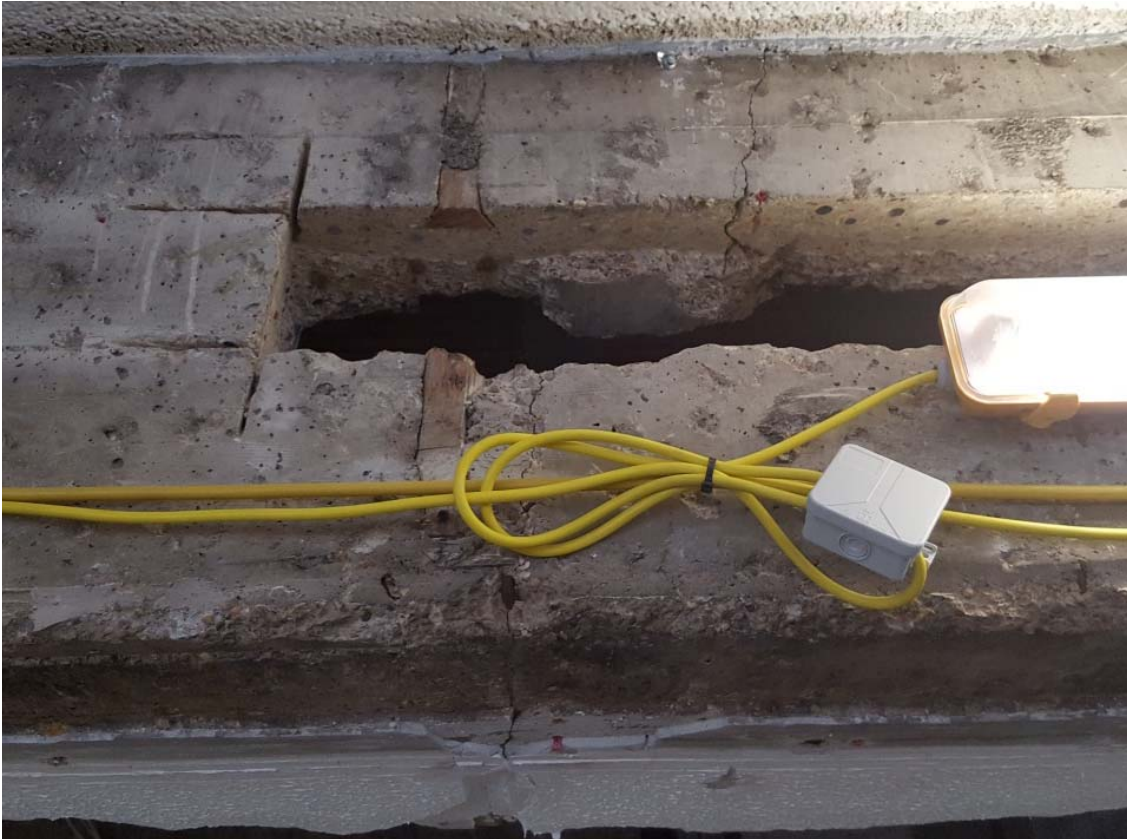
Plate 6 – View onto large service hole depicting vertical cracks in the remaining concrete (1)
