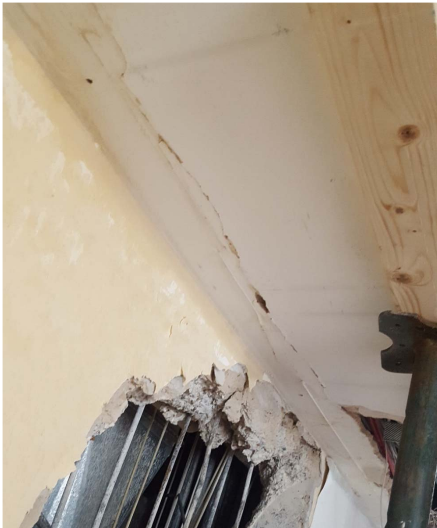
Plate 2 – View onto underside plenum slab showing parallel crack
