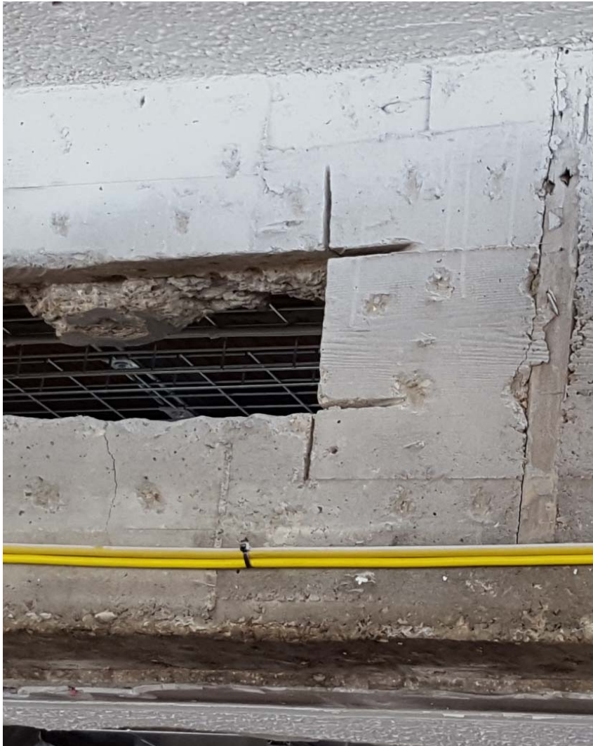
Plate 5 – Typical overcutting of large service hole
