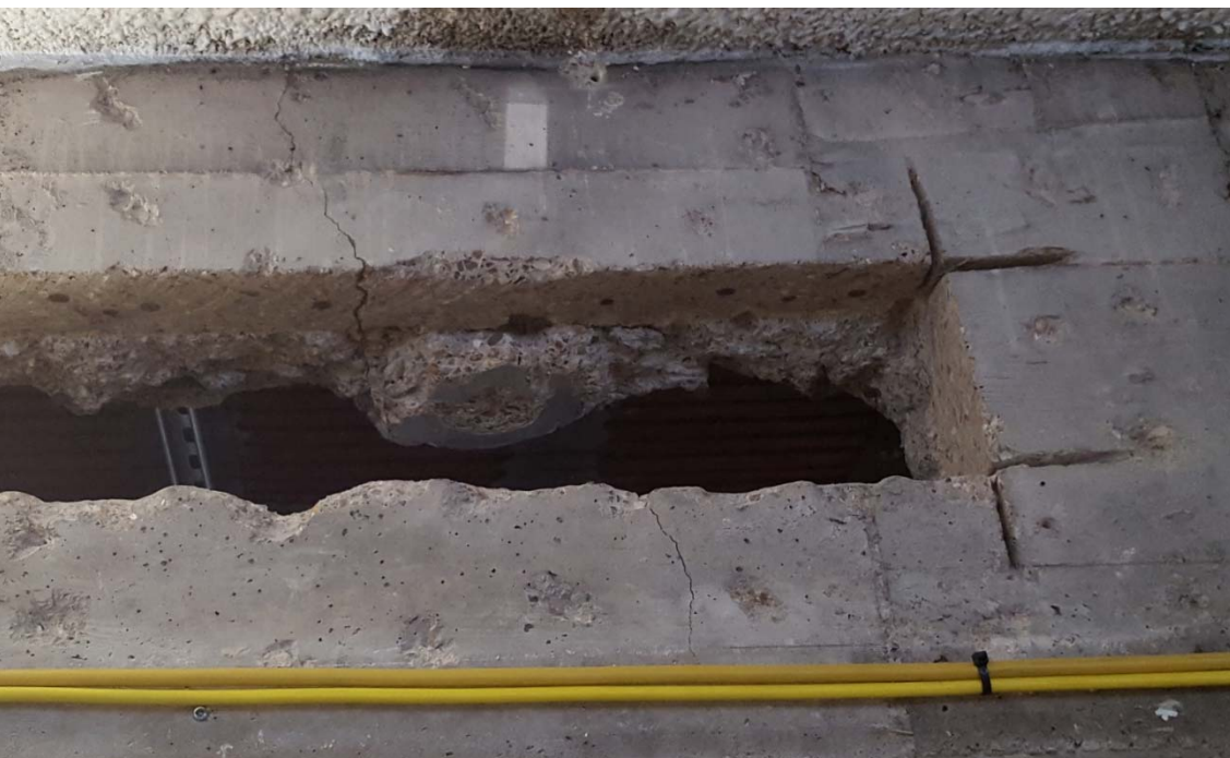
Plate 7 – View onto large service hole depicting vertical cracks in the remaining concrete (2)
