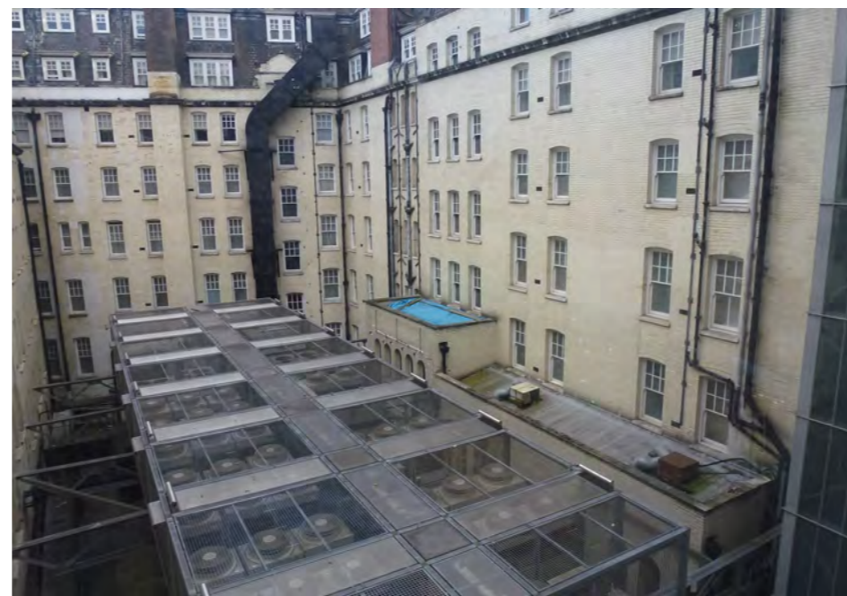
Figure 17: View of the Hotel's inner courtyard where a network of modern mechanical plant elevated above.
