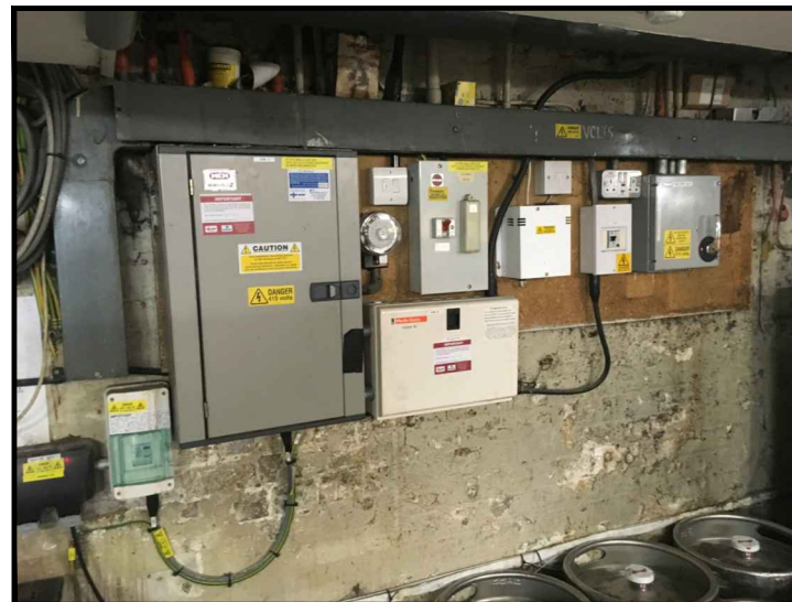
EXISTING SITE PROVIDER DISTRIBUTION BOARD
