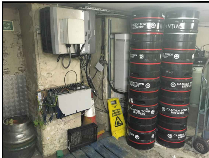
VIEW A – PROPOSED 27U RACK LOCATION, EXISTING REF EQUIPMENT TO BE REMOVED/RELOCATED
