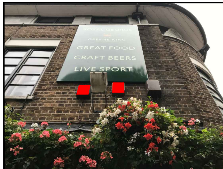
EXISTING ANTENNA A1 & A2 TO BE REPLACED
