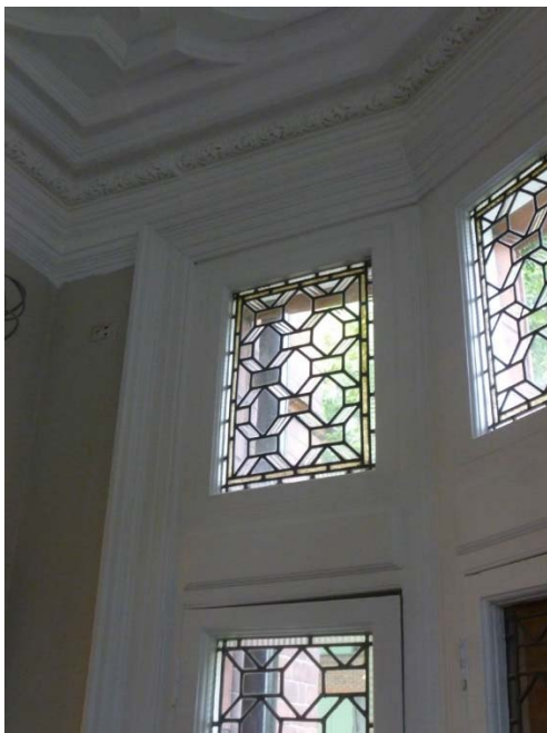
Head rail to be fitted on transom. Raised panels to be retained and protected.
