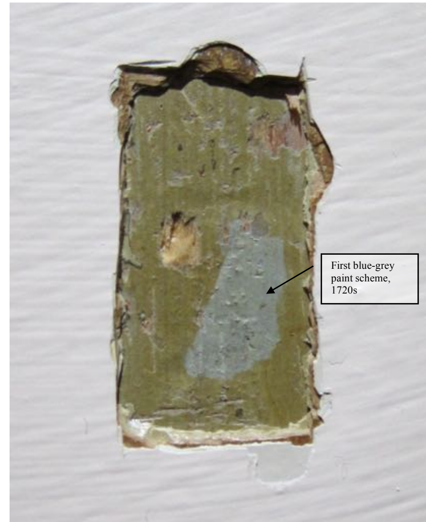
Figure 4: Uncovering on the west wall panelling, revealing the first blue-grey oil paint scheme below numerous layers of later paint. (Newly-exposed areas of original paint have a greenish appearance due to pronounced yellowing of the oil binder when not exposed to sunlight.) Uncovering ~10mm wide.
