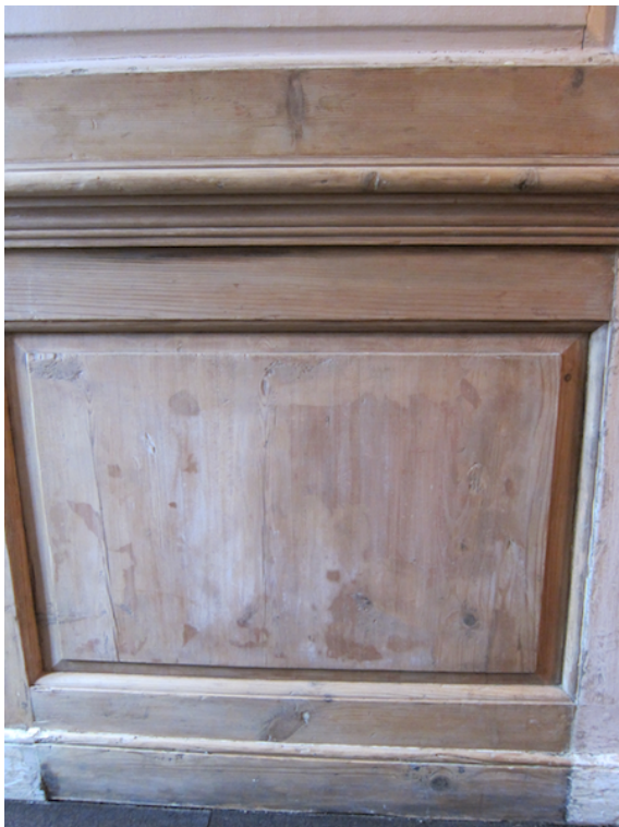
Panelling after paint removal, all paint removed, requires sealing and waxing/polishing to improve timber finish.
