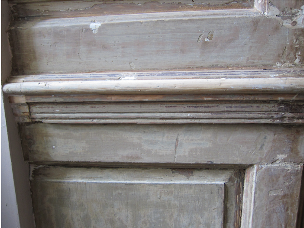
Left panel with removal of modern layers only, lead oil paints remain exposed
