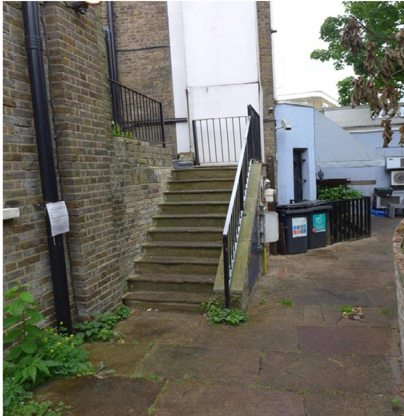
View of rear access steps to flats where gate will be positioned between side wall of steps and adjacent brick wall.
