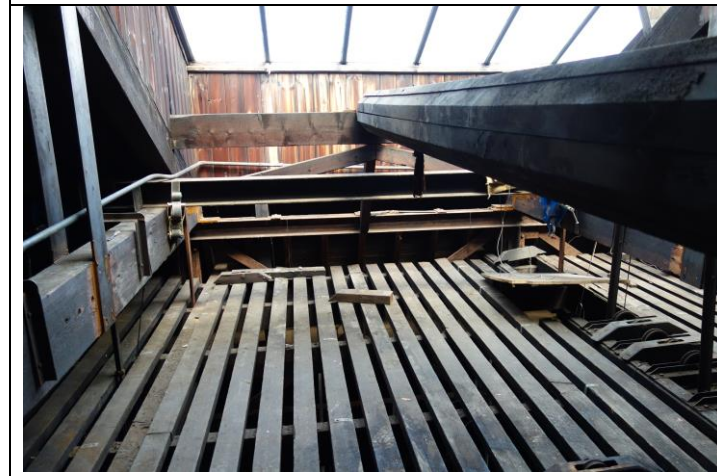
Fly tower grid
