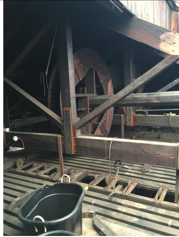
Existing original scenography equipment in the fly tower including grid and pulleys
