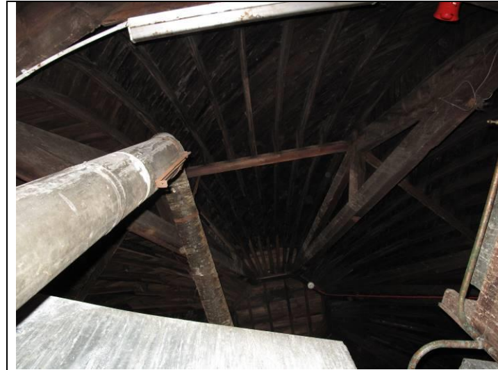
Inside of the original copper dome. The duct is probably the heat extract from the early film projectors.
