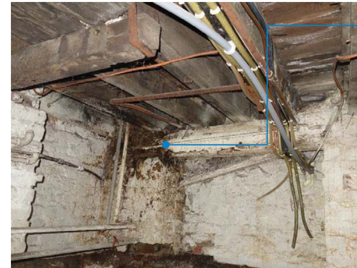
1.3 Water damage and rotting ground floor timber joists and supporting timber lintel (location B21).
