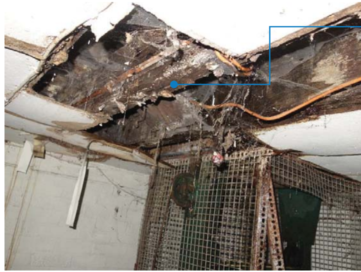
1.6 Water damage and rotting ground floor joists (location B24).
