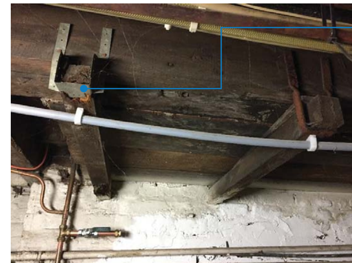
1.4 Existing timber beams supporting ground floor hearth in poor condition, with timber crushing at the joist hanger (location B21).
