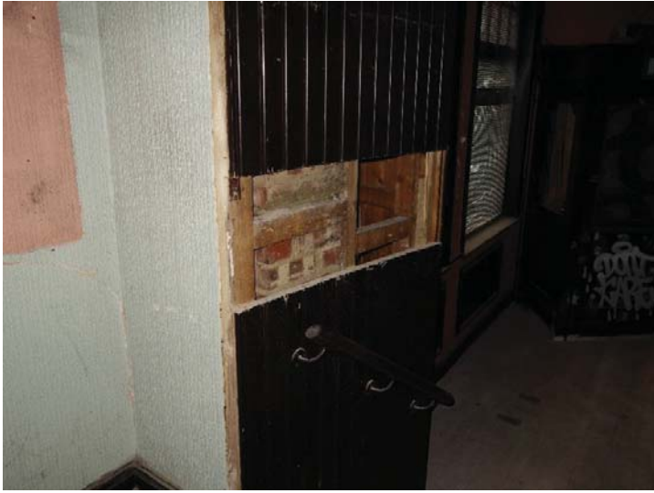
Brick piers exposed behind wall finishes (location G18).
