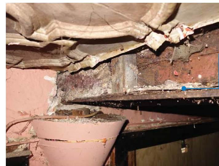
2.4 Steel beams supporting flat roof (location G19). Steel angles connected to the beam flange supports a concrete slab (filler joist concrete slab assumed).
