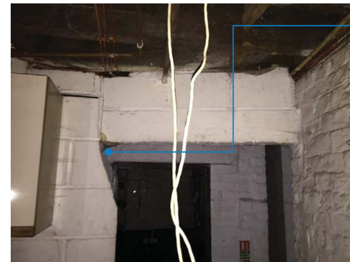
1.5 Loss of support to existing block lintel.
