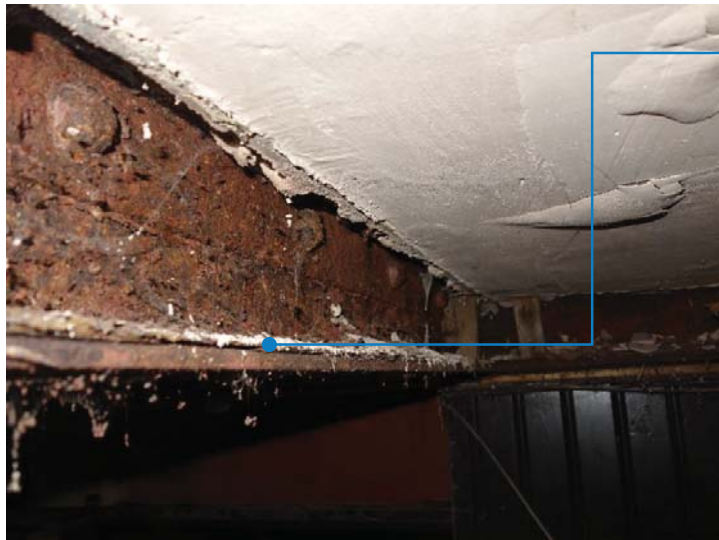
2.6 Corrosion of flat roof beam bottom flange.
