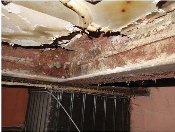
2.5 Steel beams supporting flat roof. Steel angles connected to the beam flange supports a concrete slab (filler joist concrete slab assumed). Beam bottom flange has suffered significant corrosion.
