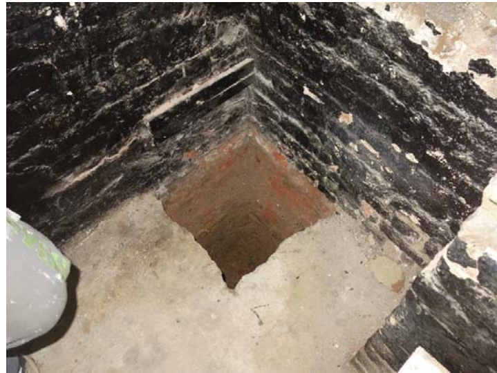
1.1 Trial pit exposed load bearing masonry bearing directly on clay approximately 400 mm below existing slab level (location B23)
