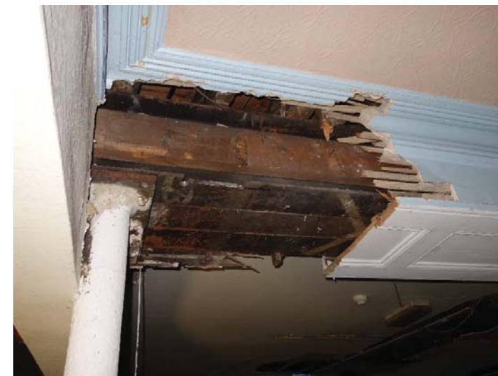
2.3 Triple steel beams measured to be 300d x 155w each (location G16). Comparison of the measured dimensions with the rolled beam sizes by Dorman Long & Co (1887) indicates the beam may be an imperial size 12x6x57.
