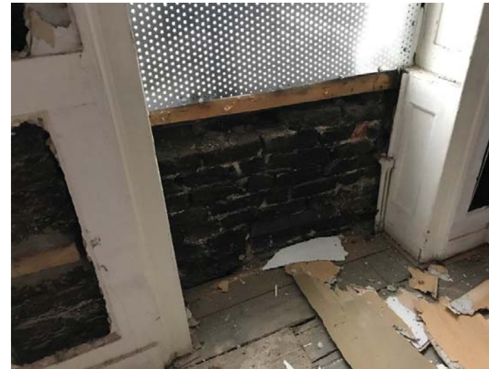
3.4 Poor quality brick and mortar in existing façade walls, particularly in spandrel panels.
