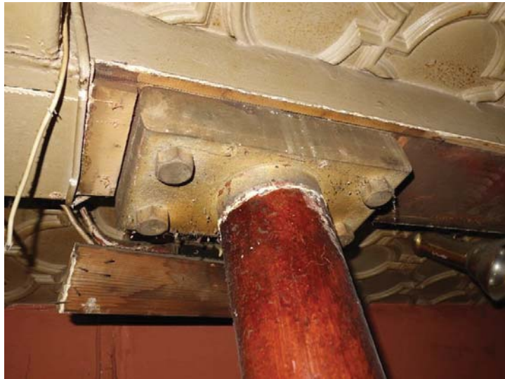
2.7 Thick top plate connection of cast steel post to steel roof beam (location G20).
