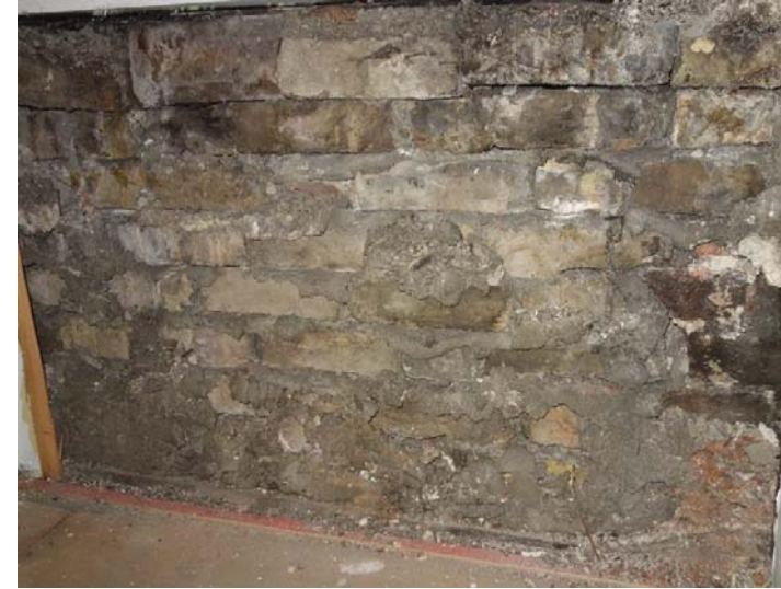
3.3 Poor quality brick and mortar in existing façade walls, particularly in spandrel panels.
