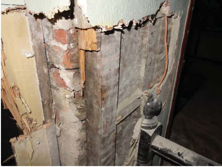
Cast steel or iron post uncovered in front of brick pier (location G17).
