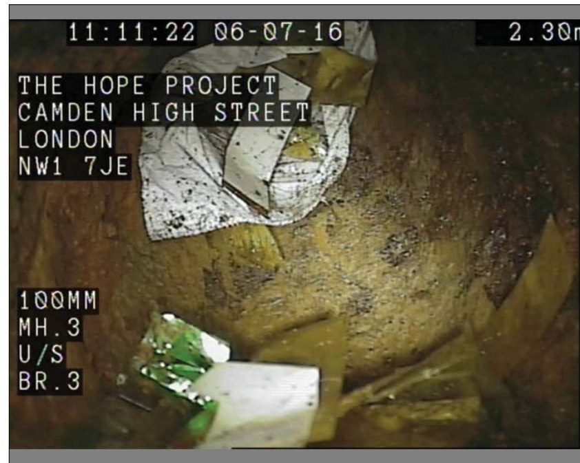
Photo: 9_9_44_A.JPG 2.3m, Settled deposits, coarse, 80% cross-sectional area loss
