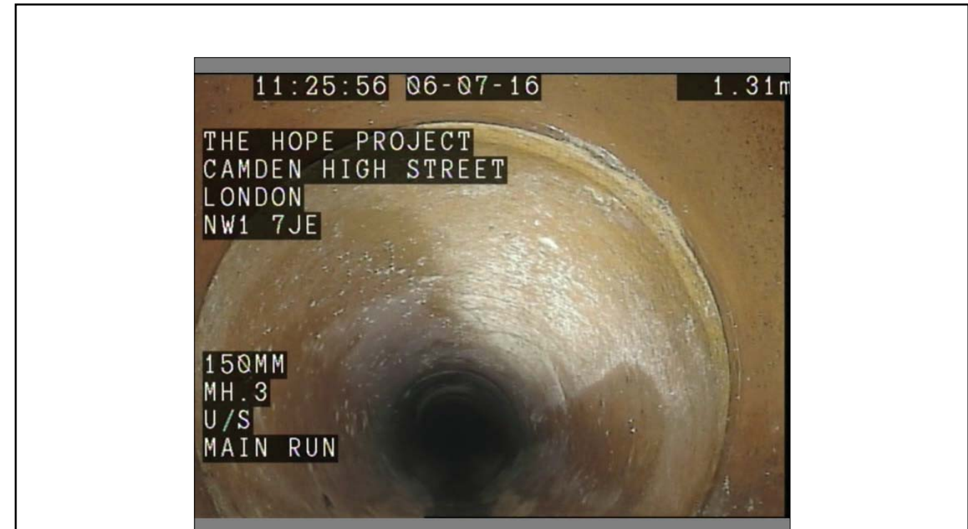
Photo: 12_1_6_18072016_124539_A.jpg 1.31m, Crack, circumferential at joint, from 1 to 4 o'clock
