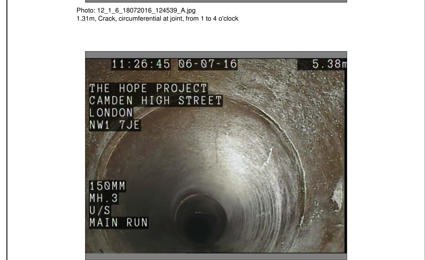
Photo: 12_1_7_18072016_124600_A.jpg 5.38m, Crack, longitudinal at joint, at 1 o'clock
