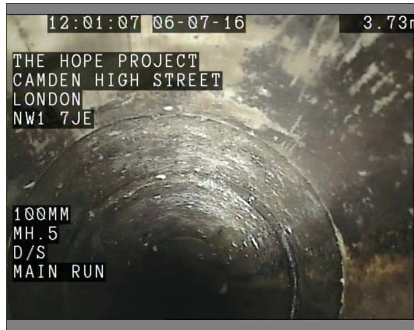
Photo: 17_17_107_A.JPG 3.73m, Crack, circumferential, from 7 to 4 o'clock
