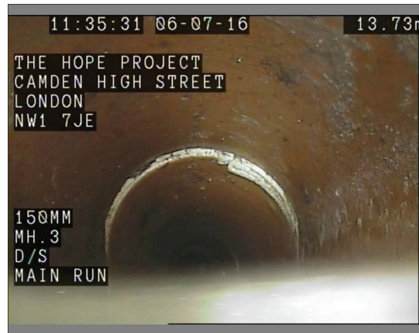
Photo: 14_14_82_A.JPG 13.84m, Broken pipe at joint, from 1 to 3 o'clock
