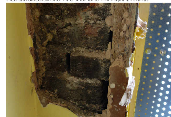
Poor condition brickwork in The Hope & Anchor
