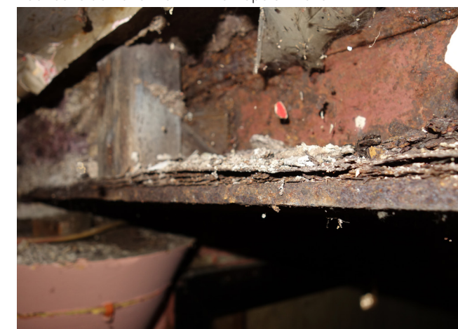
Corroded steel roof beams in The Hope & Anchor
