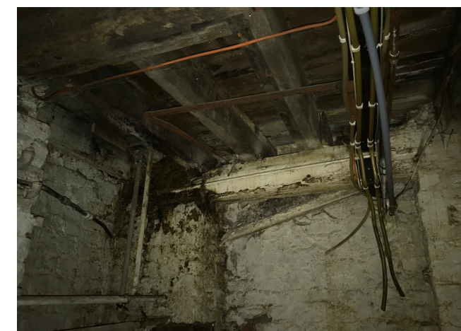
Poor condition timber beam in The Hope & Anchor
