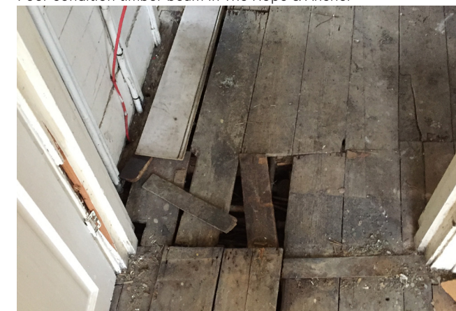
Poor condition timber floor boards in The Hope & Anchor
