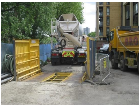
Typical Recycled Water Wheel Wash Facility
