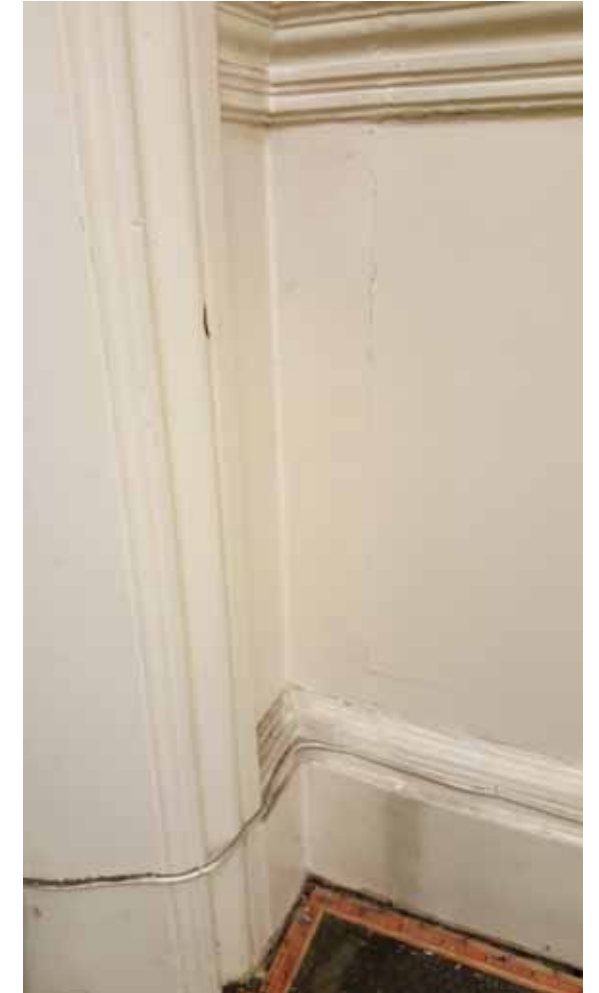
Where the front wall meets the party wall, a crack can be observed about 4 inches in from the corner on the party wall side. This extends through the dado and the skirting elements indicating that these details were extended following the removal of the 'false' wall that was associated with the shutter boxes.
