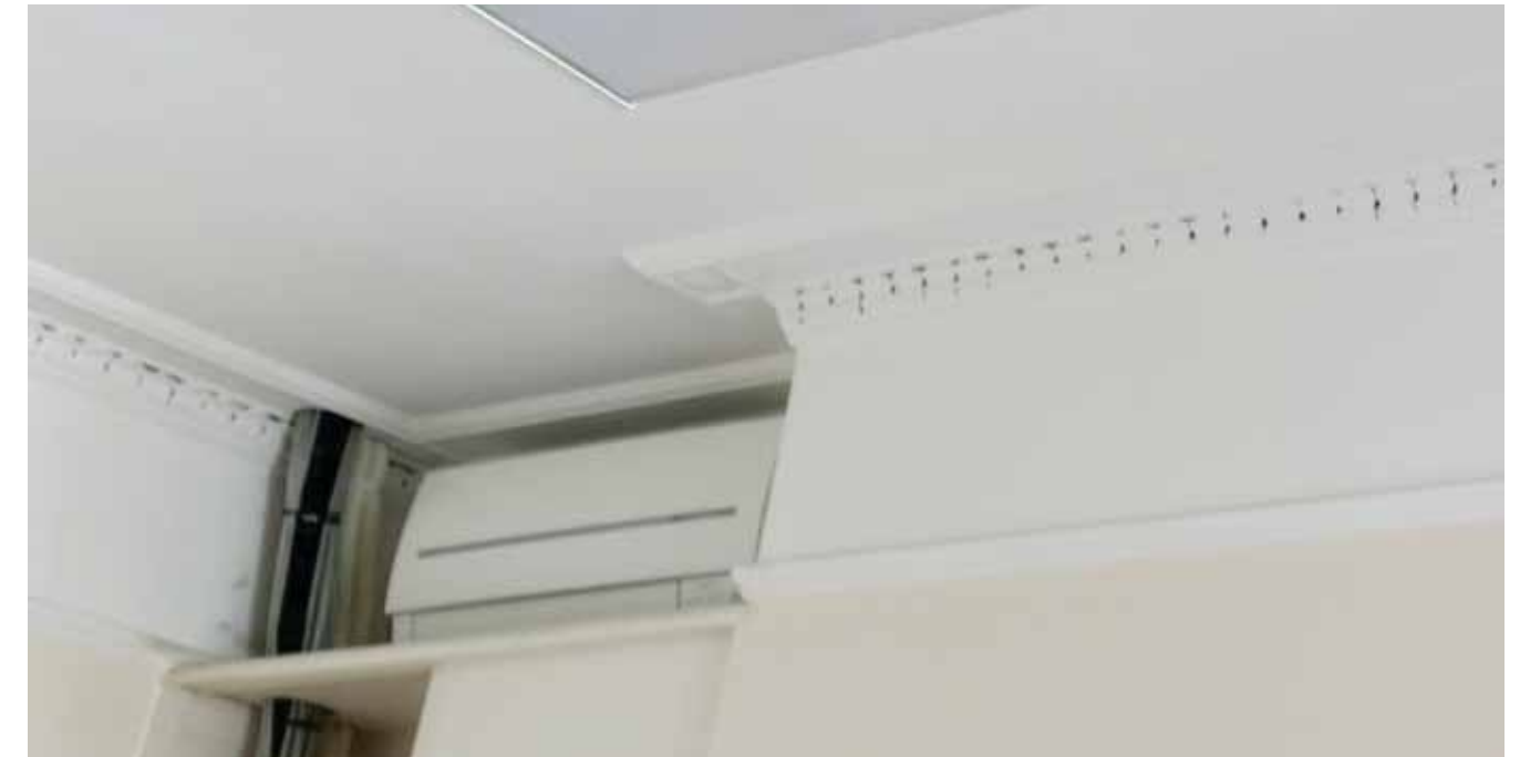
Original cornice feature though with some recent thoughtless damage.
