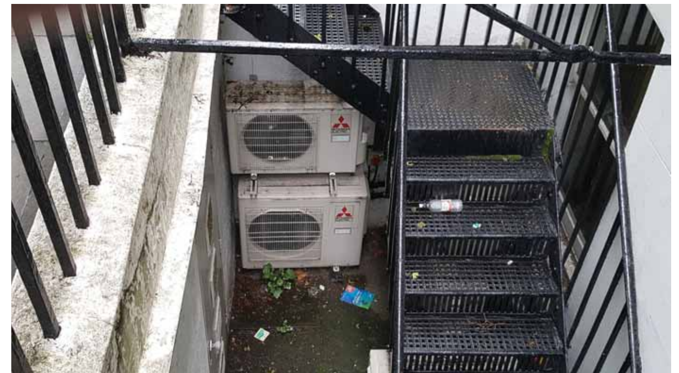
The front light-well. A cast iron stair in place of what would have been a stone stair. 3 fan coil units serving the air conditioning units within the offices.
