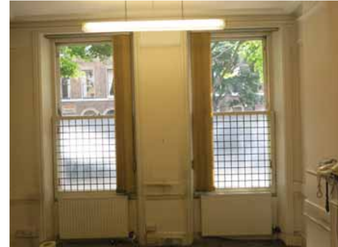
Edwardian 1-over-one sliding sashes, without shutters. Obtrusive privacy glazing has been installed over the lower half. The thick Edwardian cornice which has a haphazard relationship to the window architraves.
