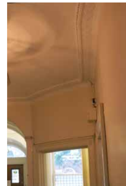
Hallway cornice against wall to R0-3 gently curved in to allow enough space for door to R0-1.
