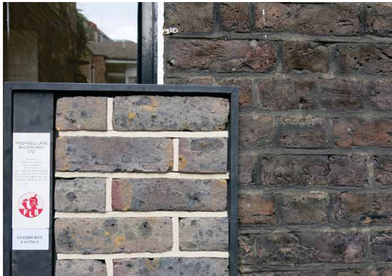
Photograph taken on site at rear on no 42 showing sample panel of 'Overburnt Facings' bricks by Freshfield Lane Bricks, alongside the existing brickwork. The tones of the bricks are relatively close to one another. A similar coloured mortar will be used for the pointing of the existing wall and laying of the new wall.
