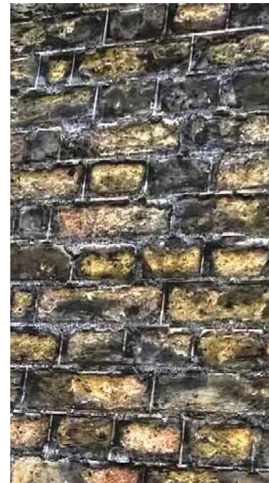
Extract from Report on Decay and Remediation by Terrence Lee (Appendix E). In places it can be seen that the spalling to the brick faces is quite severe at no 42.
