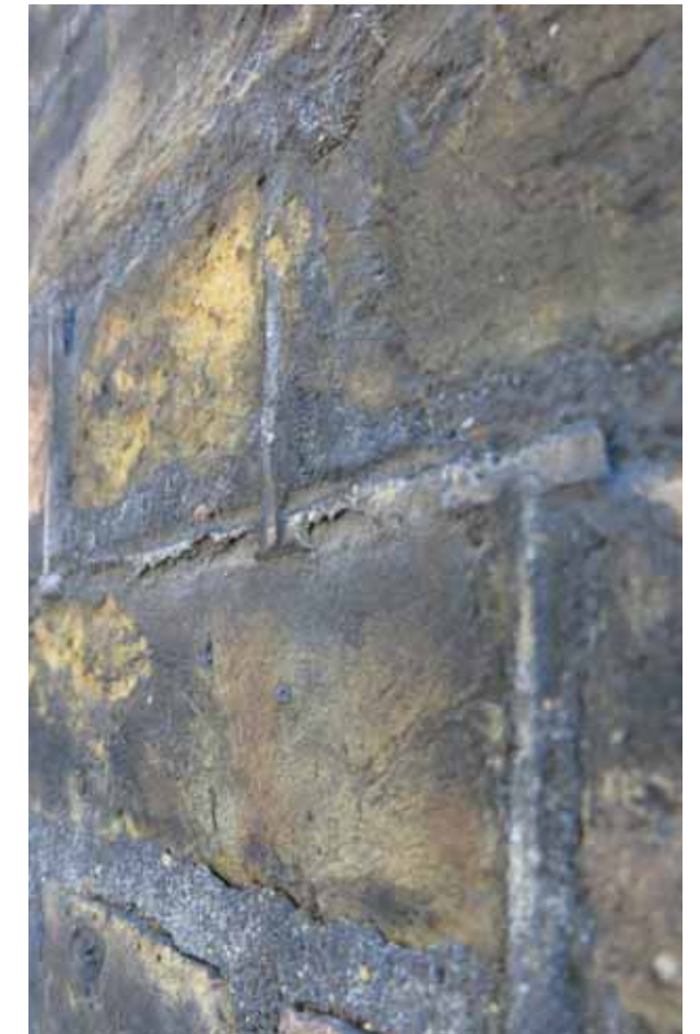
Close up of brickwork at ground floor at no 42. The dark stopping mortar has gaps between it and the bricks in places which is likely to be encouraging excessive wetting during rainy periods. This in turn may be accelerating the spalling.
