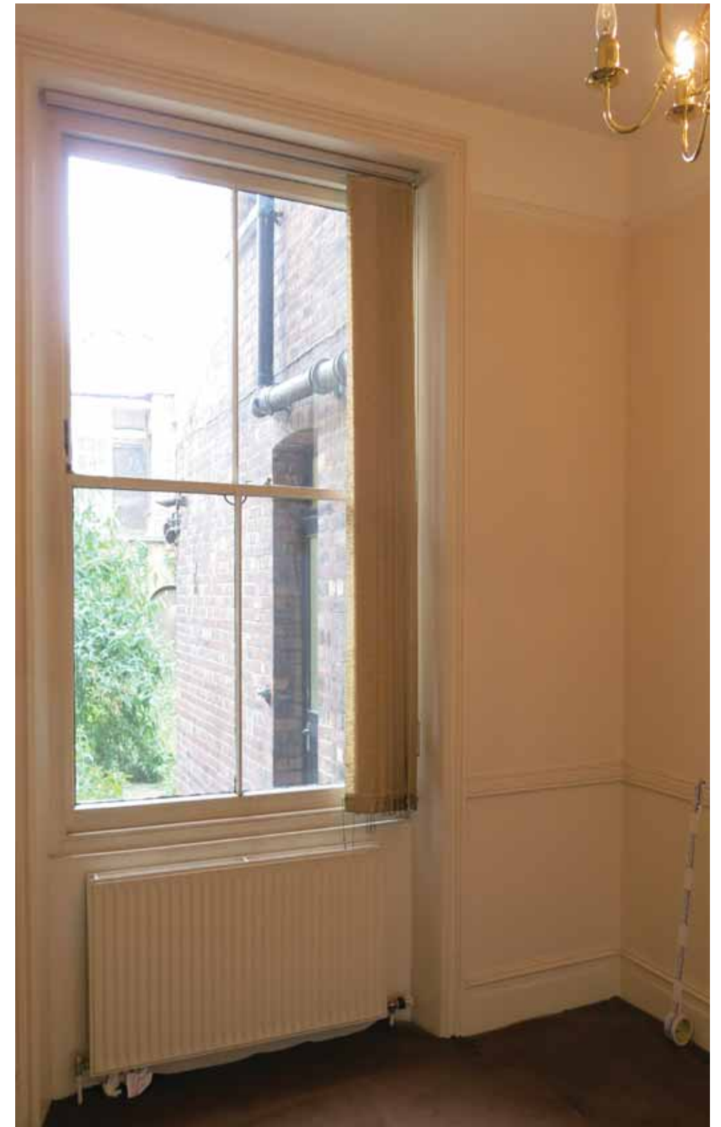
Edwardian sash window and loss of shutters, false wall, cornice and original skirting and dado.
