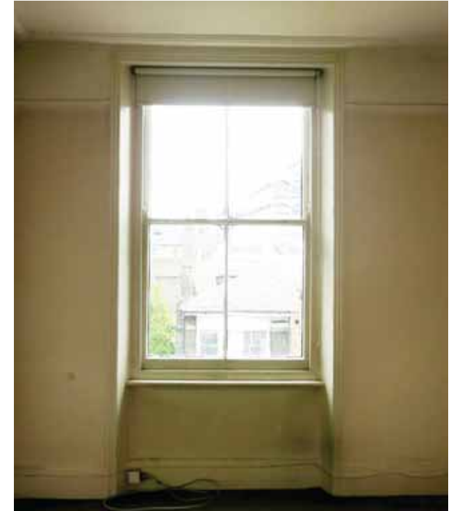
2 over 2 Edwardian window with missing window apron shutters and false wall.
