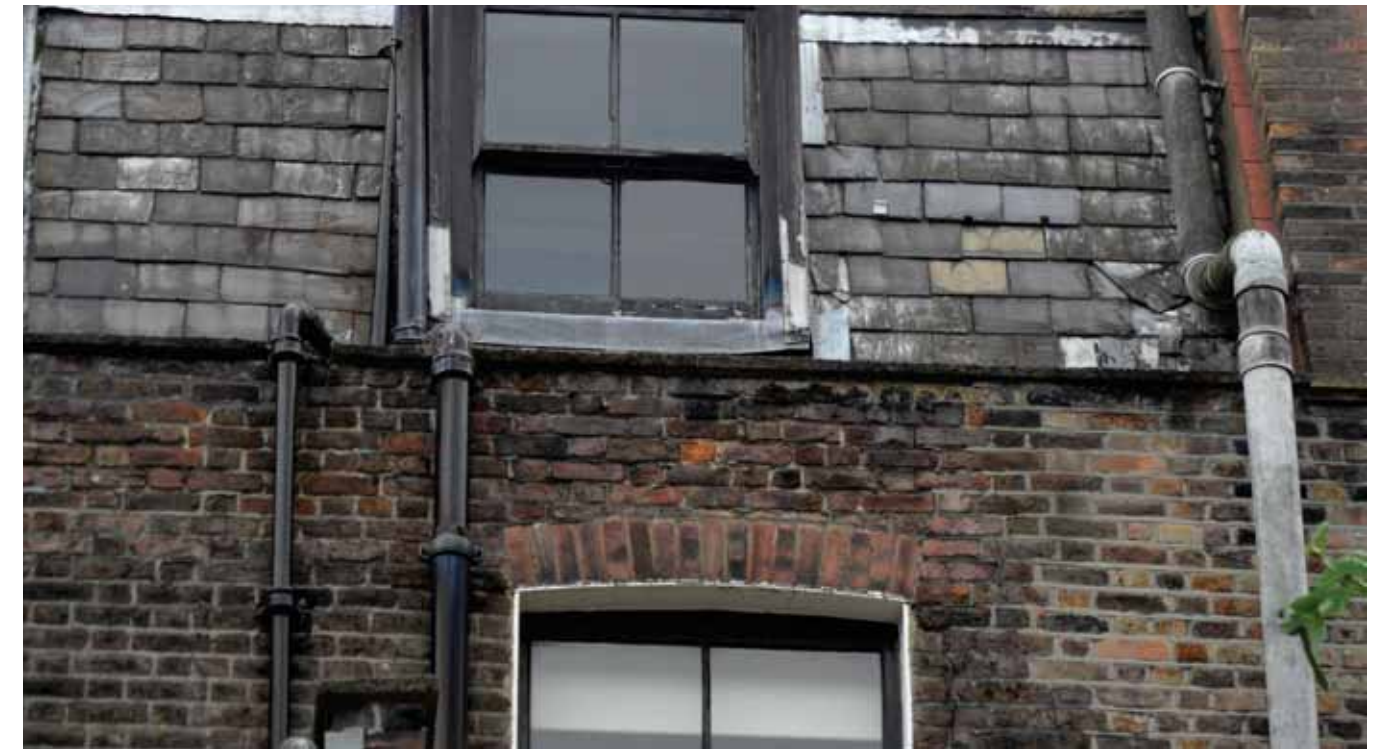
The upper parts of the brickwork to the rear facade which show signs of loss of pointing and brick damage as a result of failed coping stones. The repairs to the right hand side of the picture appear to have been executed in inappropriate cement.
