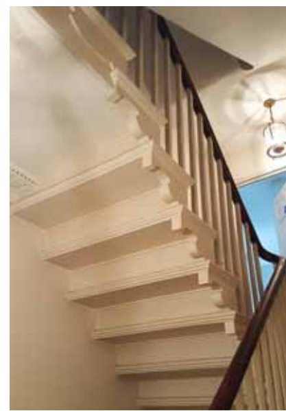
'Cantilevered stone' affectation in timber. Highly unusual.
