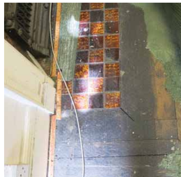
The original stone hearth has been reduced in size and replaced with glazed tiles.
