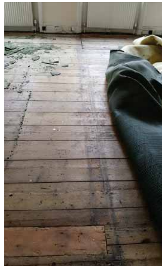
Mark on floor from previous partition wall.
