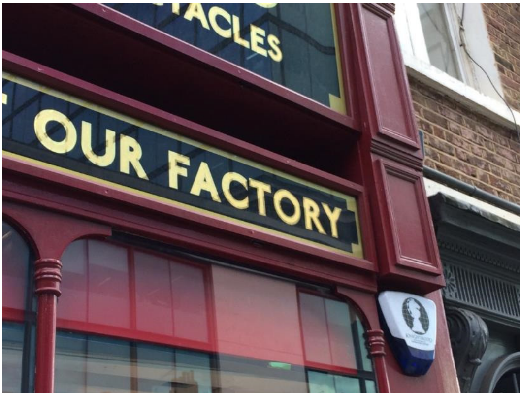
Photograph of existing recess within timber shop front joinery for the awning.
