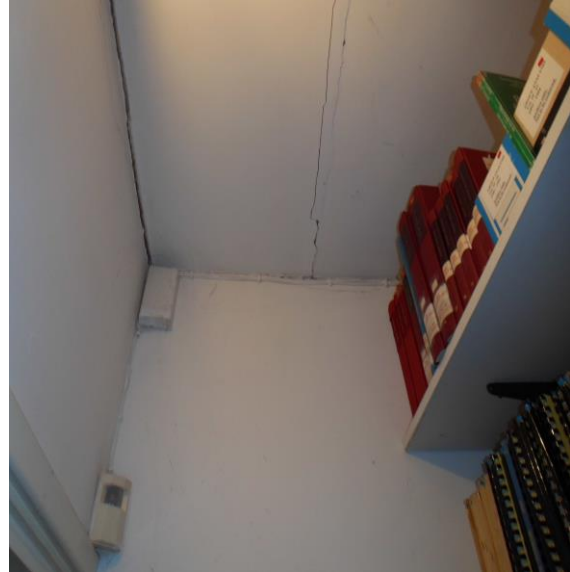
Ceiling crack to library cupboard
