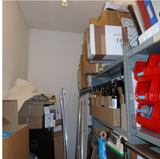
Fracture to partition wall to cupboard no. 23
