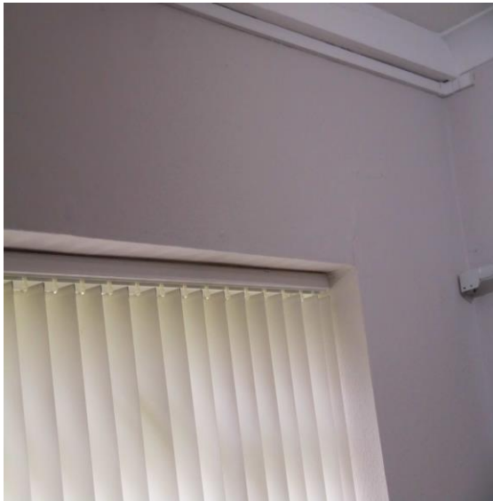
Rear meeting room crack above right of window
