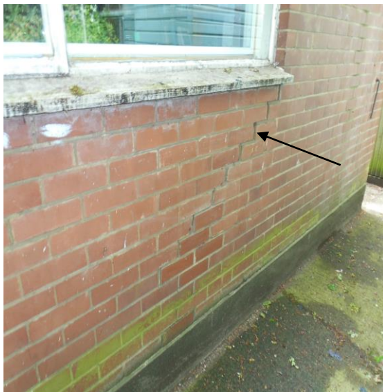
~Stepped diagonal crack below window along flank wall to library
