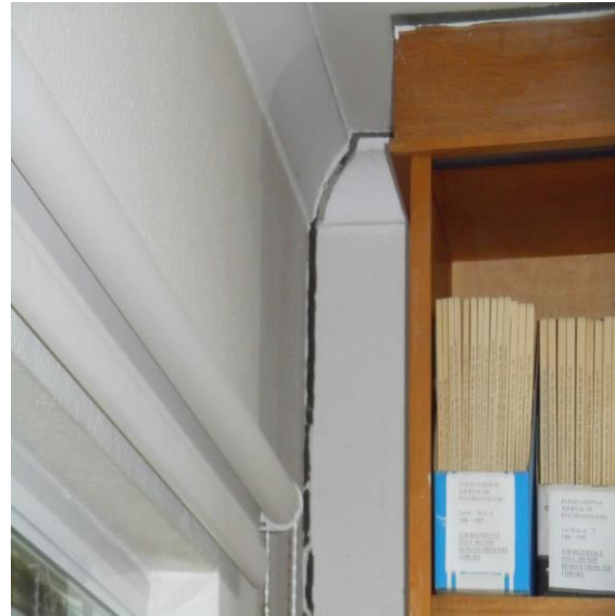
Close up of crack to right of window in the library
