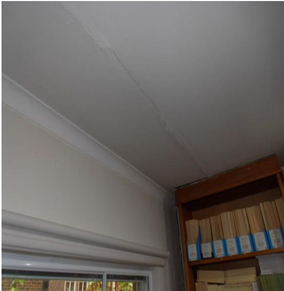
Library ceiling crack to rear of room
