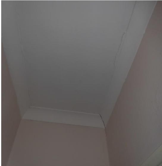
Ceiling crack in corridor near library
