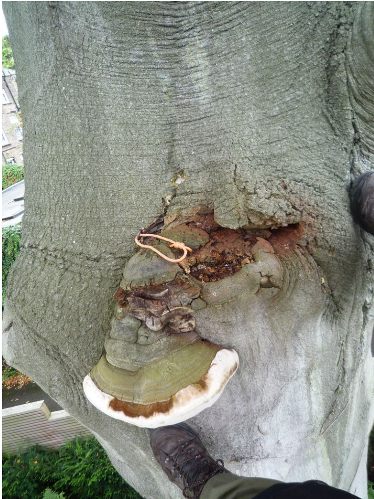
3) Ganoderma bracket at 6m, below smaller, older brackets. Note large open wound and the end of a 400mm long probe with orange loop.
