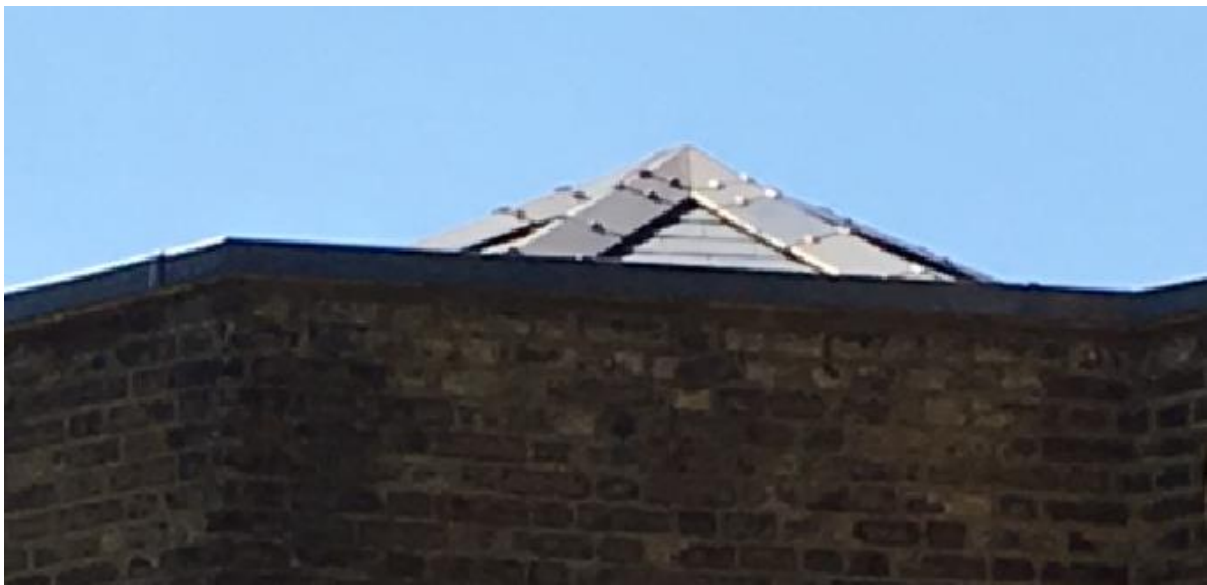
The unauthorised ridge fixings
