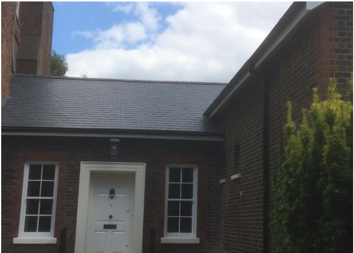
The roof with the recent installation of Del Carmen natural slate and roof clip fixings
