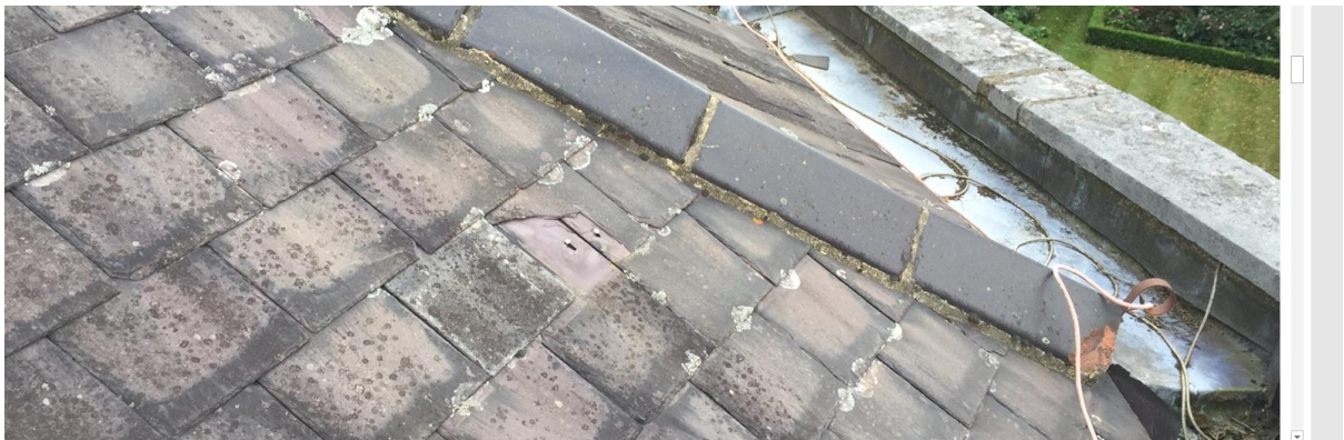
Two photos of the roof of No. 1 The Old Hall before the recent work was carried out
