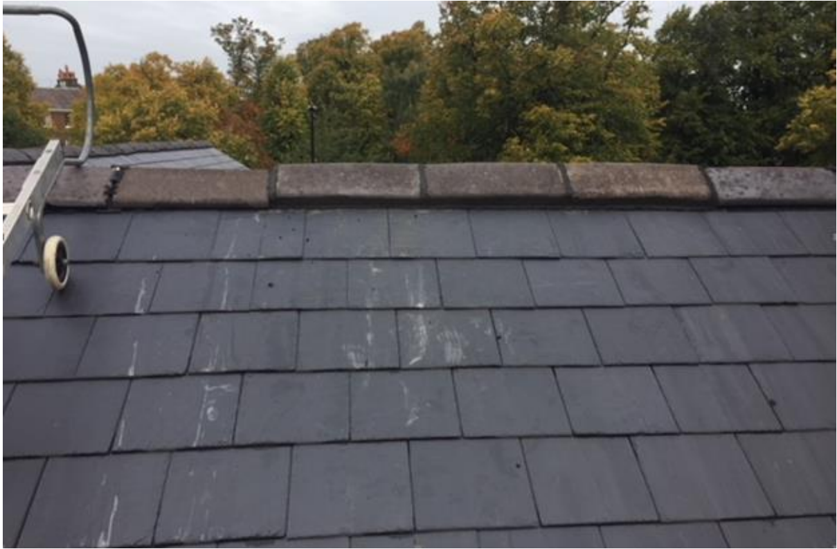
Newly laid natural Del Carmine slate tiles and on the right 4 ridge tiles re-laid in tinted mortar.
