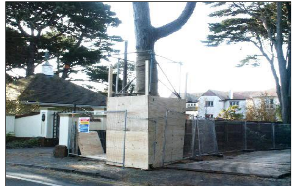
Fencing image 6: Board secured to scaffold framework adds another layer of protection for vulnerable trunks and branches
