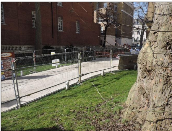
Ground protection image 1: Poured concrete slab outside of tree protection fencing creating an access route into the site.
