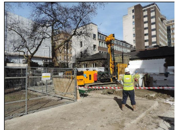
Ground protection image 2: Small piling rig operating whilst standing on concrete ground protection.
