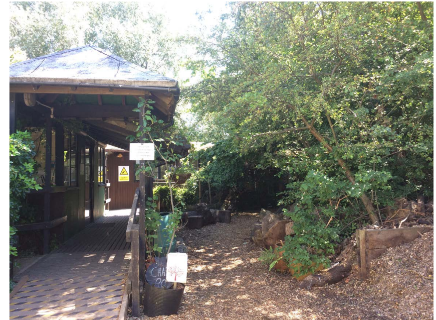
③ view of ramp, handrail, side wall of volunteer room and canopy to be demolished
