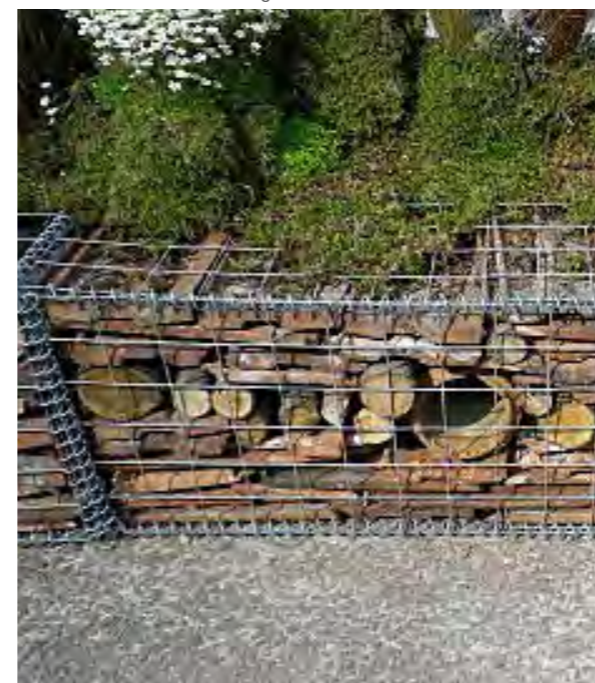
Example of gabions filled with habitat features and working as a retaining wall
