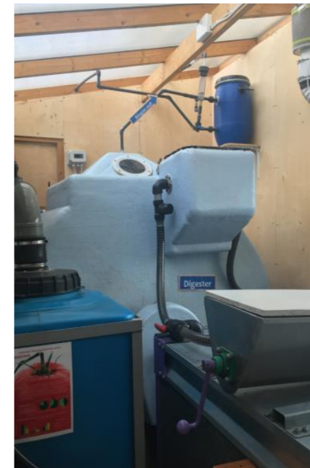
⑩ anaerobic digester system to be removed to be reused at another site (main digester and associated plant)
