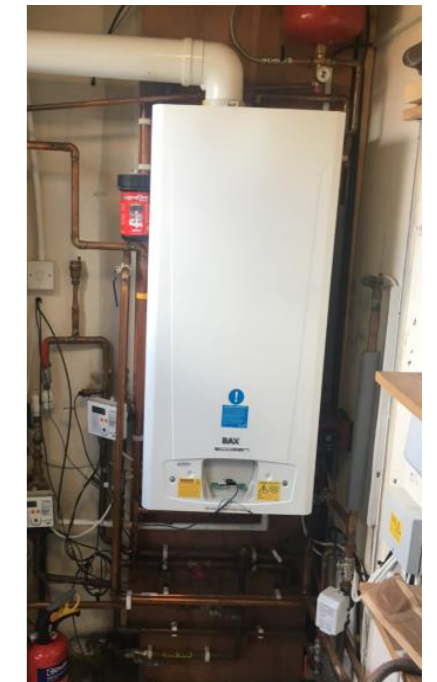
⑪ anaerobic digester system to be removed to be reused at another LWT site (micro combined heat & power unit)
