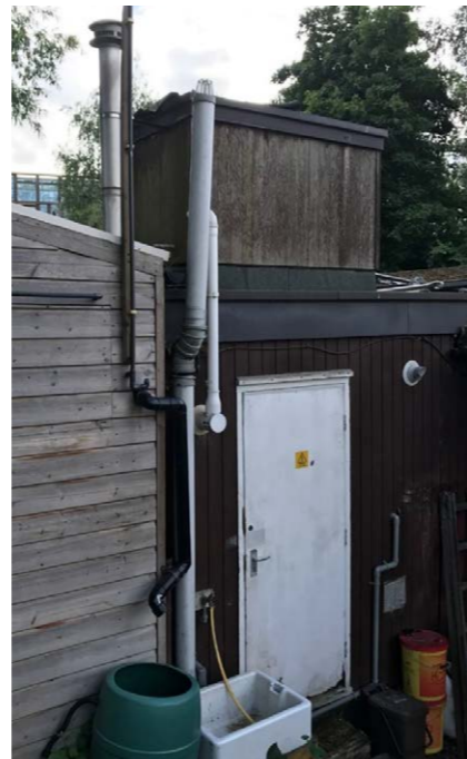
⑧ existing boiler room showing flues, water recycling and roof mounted water storage tank to be demolished
