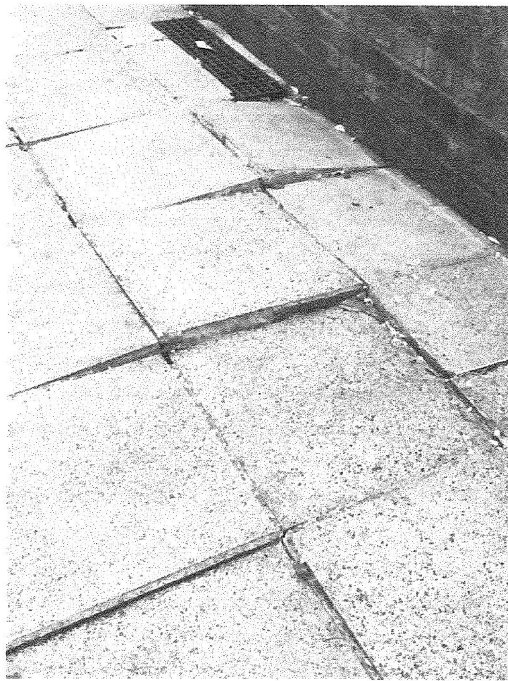
pictures of damage caused by Cherry roots to garden wall & patio
