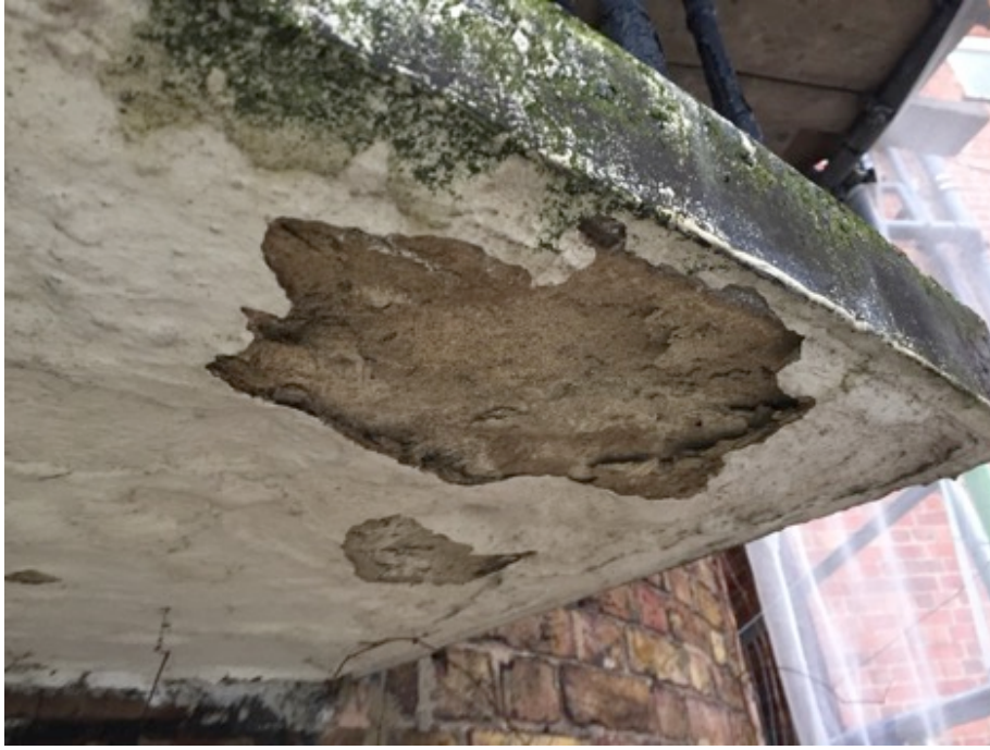
Photograph 3 – Large section of the underside of balcony fallen off
