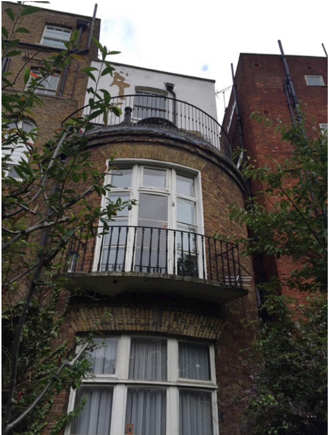
Photograph 2 – The balcony as deemed unsafe
