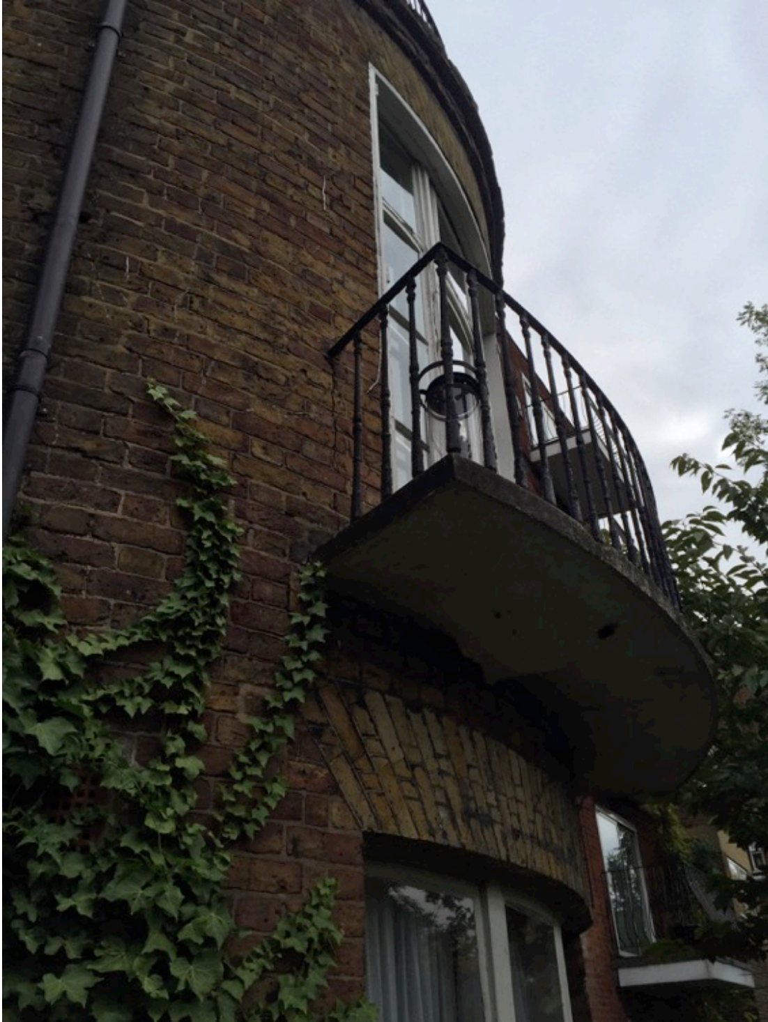
Photograph 1 – Balcony in disrepair
