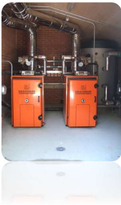
Figure 7: Communal Biomass Installation (Author's Own Image)
