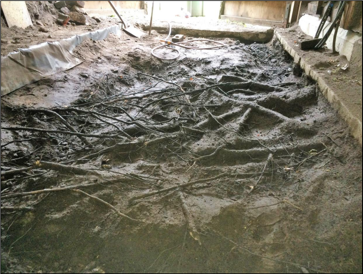
Figure 4: An example of an air spade excavation to determine the location of roots
