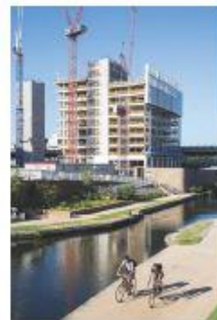
Building works adjacent Regent's canal during the construction of the King's Cross Development
