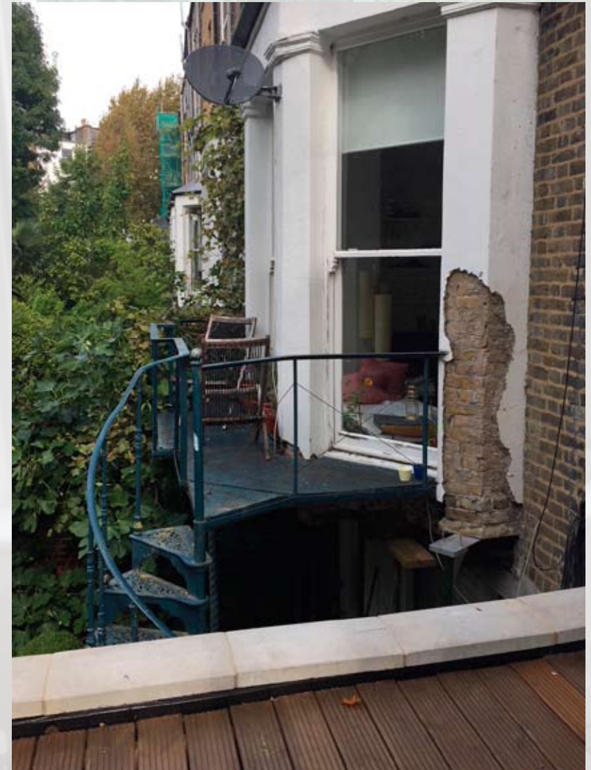
Next door terrace is in very close proximity with the existing Terrace
