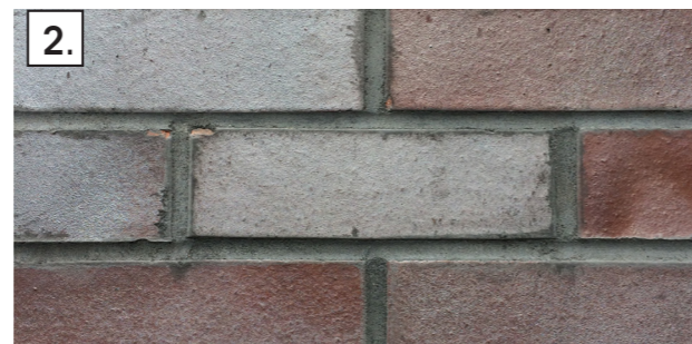
2. Brick Type 1, to Landmark Building and spine of lower blocks : Janinhoff Blue/blue red/8C
