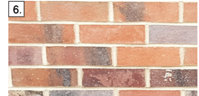
6. Brick type 2: To projecting bays on both Belsize Road and Railway elevations, Blocks A-E : STP -EF-8/Schmelzbrand
