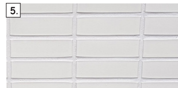
5. White glazed brick to Landmark Building Recessed balconies :Modular Clay - White Glazed brick
