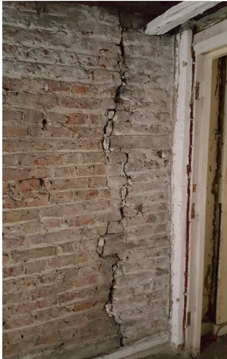
Figure 7, Typical Cracked Masonry Repair - Third Floor Party Wall Shown
