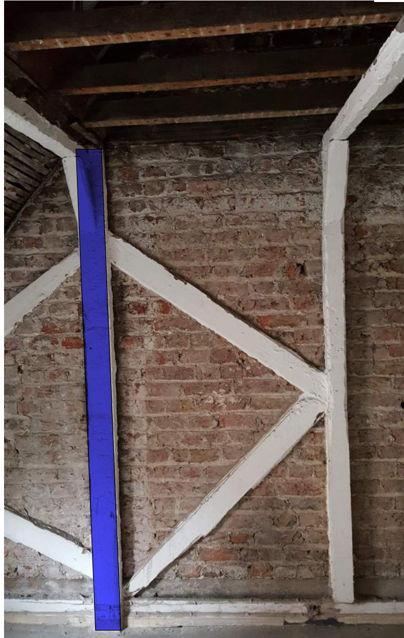
Figure 12, Third Floor Non-Structural Additions
