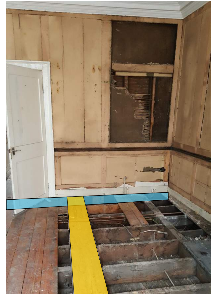
Figure 4, Floor Beam To Be Re-supported
