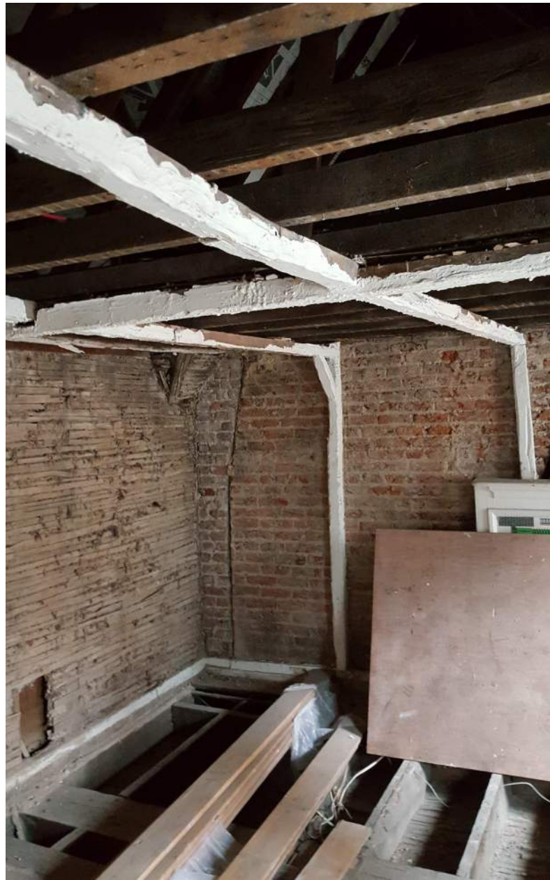
Figure 13, Third Floor Non-Structural Additions
