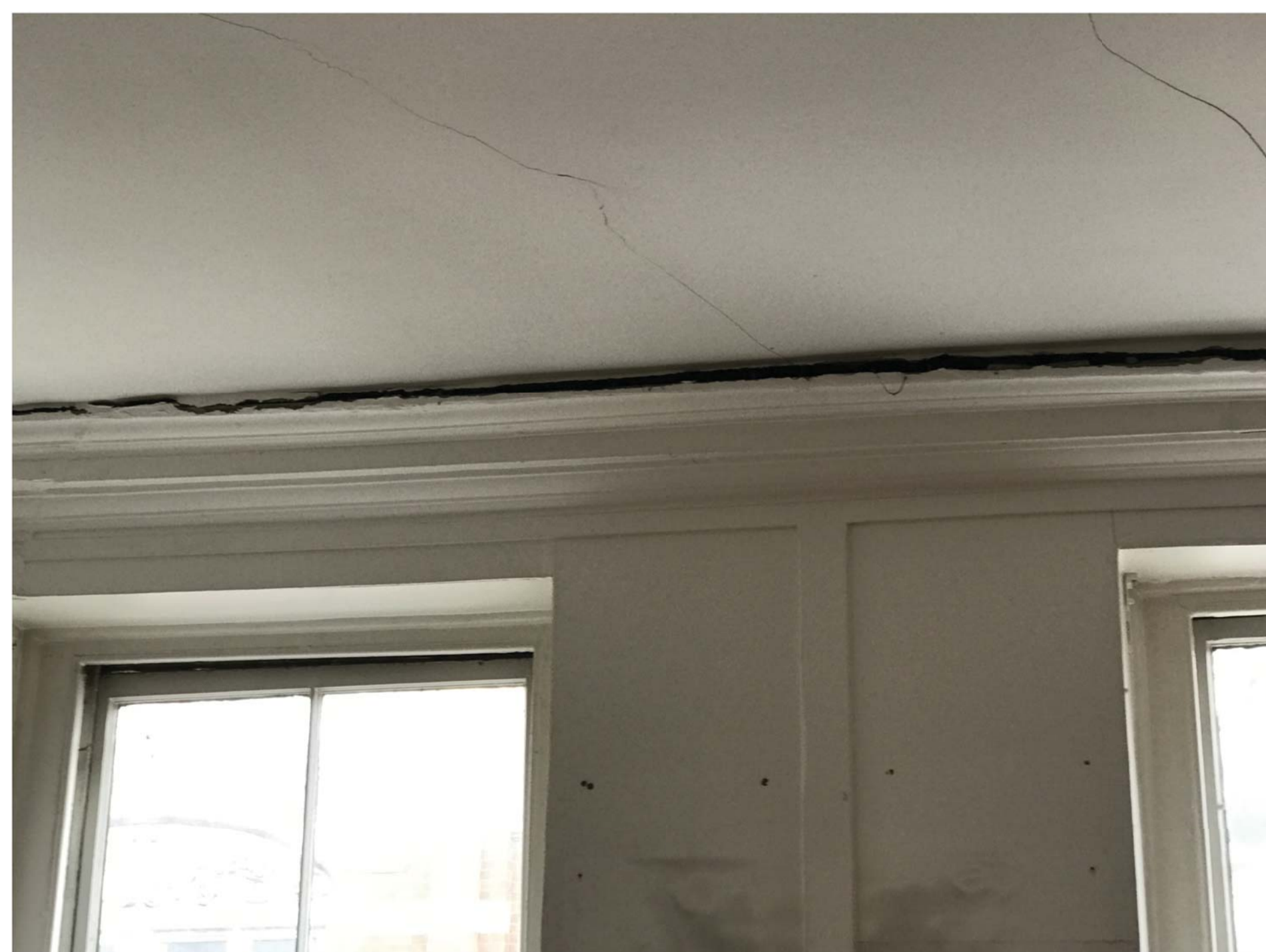
01 Existing damaged plaster cornice on second floor to be replaced X_501
