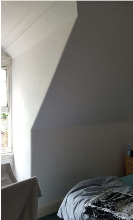
Figure 2. The internal void at the south-east corner of the building on the top floor
